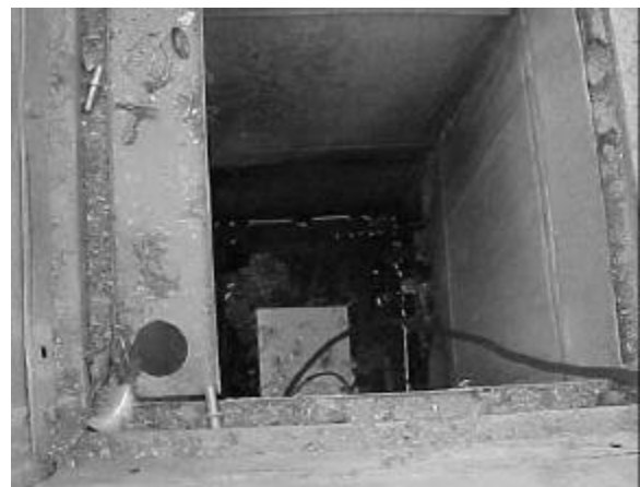
Figure 5 – Picture of regeneration exhaust viewed from roof. Water level is visible inside duct. Hose at lower right is pressure measurement reference.
