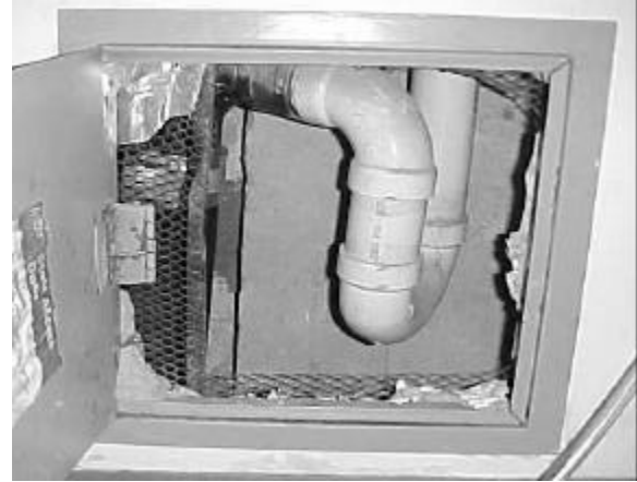
Figure 8 – Plumbing access panel that allows exhaust fan to depressurize archive.
