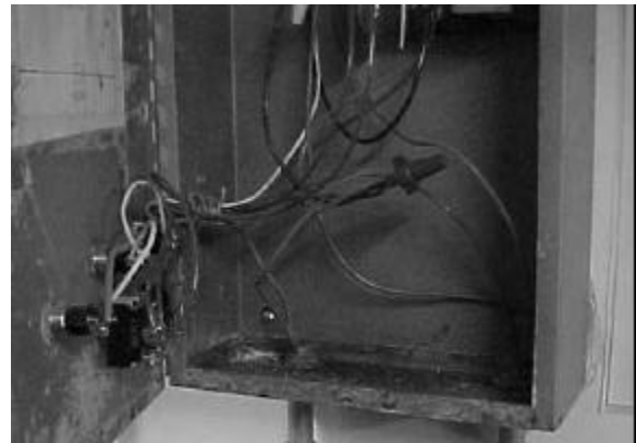
Figure 7 – Control box corrosion indicating it had been filled with water to top of door flange.
