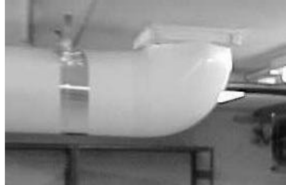
Figure 4 – Visible picture of regeneration air inlet from inside archive. Water damaged materials were found on shelves in background. This is the same duct as Figure 3.
