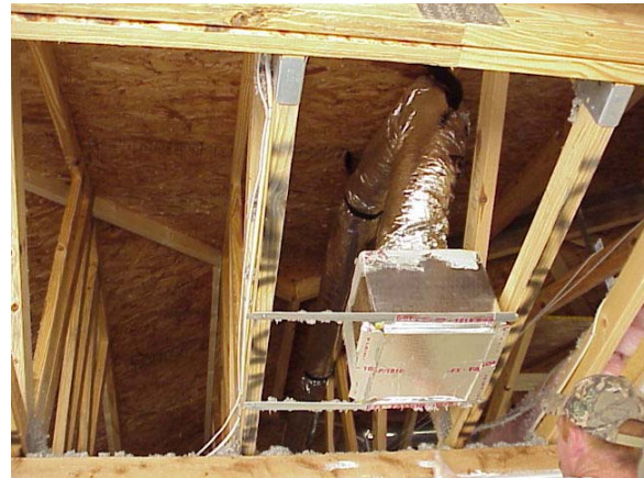
Figure 1 OA Intake Duct in Back Porch
