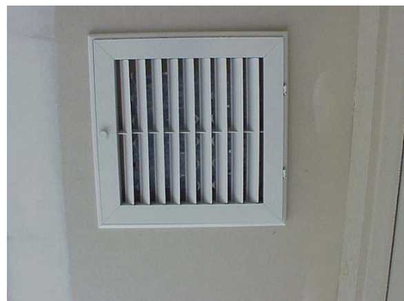
Figure 3 Filter Backed Grill Covering the OA Intake
