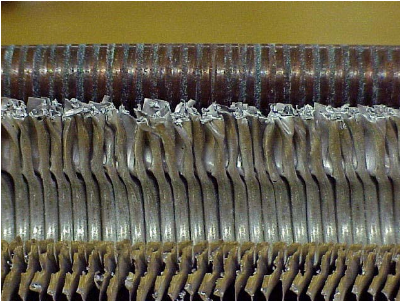
Figure 2. Corroded copper tube and adjacent aluminum fins.
