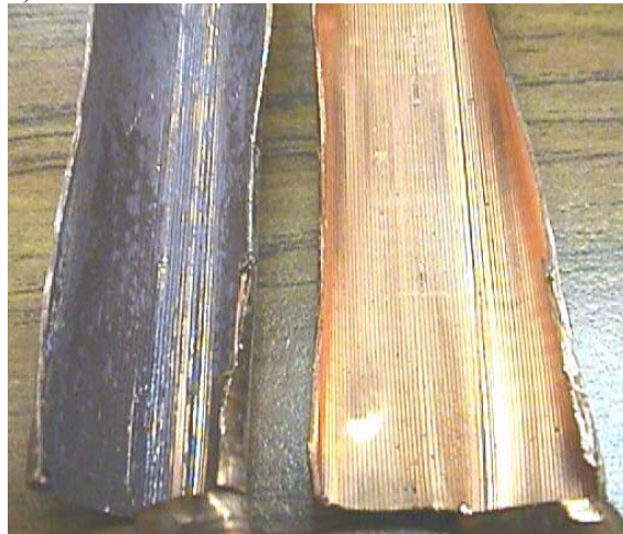
Figure 5. Interior surface of corroded copper tube at capillary inlet end (left) of circuit and at suction manifold end (right) of circuit.
