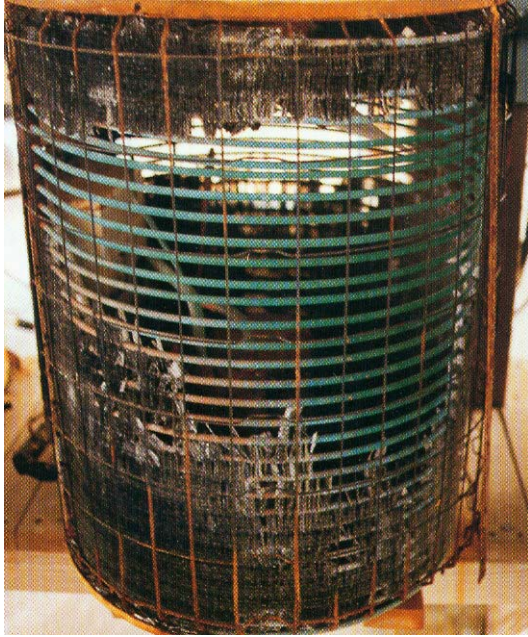
Figure 1. Outdoor Coil showing evidence of galvanic corrosion.
