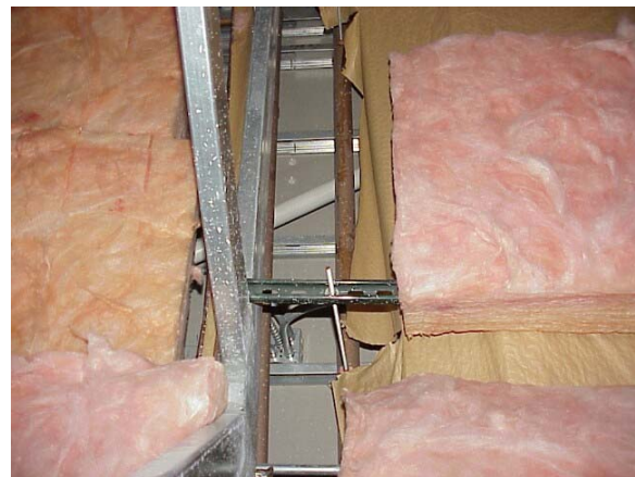
Figure 10 Typical insulation void approximately 25% to 30%.
