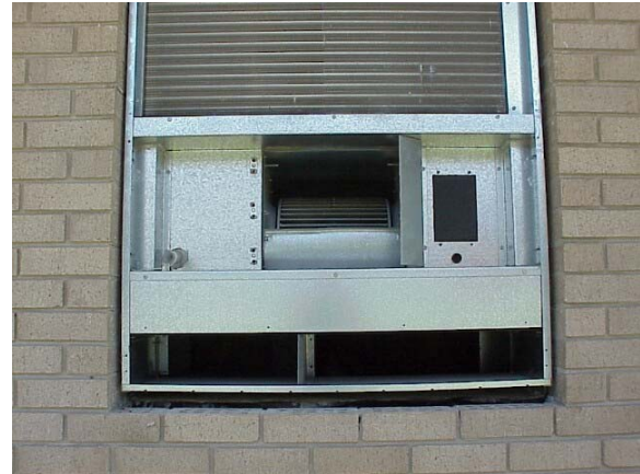
Figure 8 Exterior view of PTHP unit with grille assembly removed. Approximately 1 inch of clearance exists between the unit and the wall
