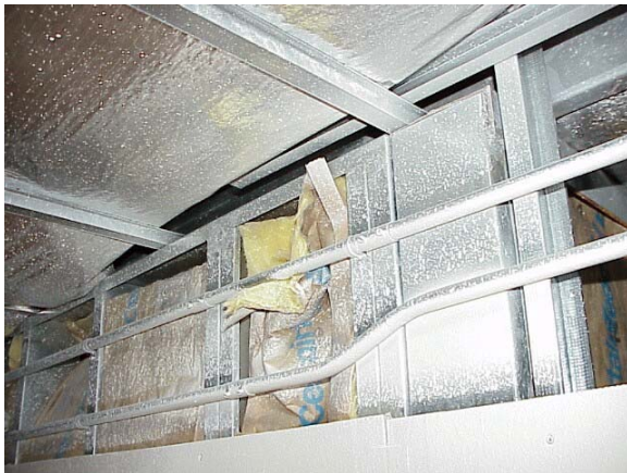
Figure 7 Incomplete air barrier at connection of wall assembly to ceiling.
