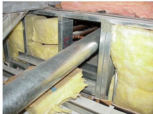
Figure 11 Vent pipe passing through the vertical wall section. Air and thermal barriers have been compromised
