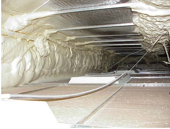
Figure 12 Attic space after foam was installed It can be seen along the bottom of the truss
