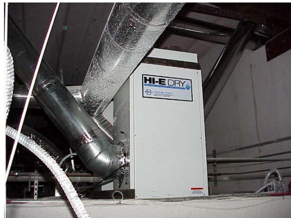
Figure 13 One of four dehumidifiers installed in the ceiling space of a quad classroom building.
