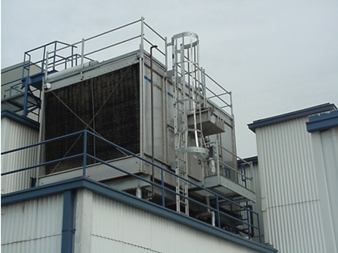
Figure 5.1. Test Facility Cooling Tower
