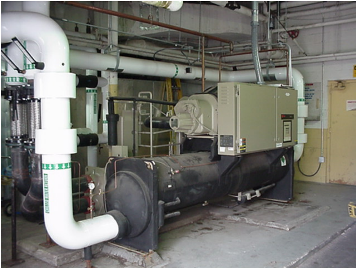
Figure 1.1. 205-ton Installed Screw Chiller
