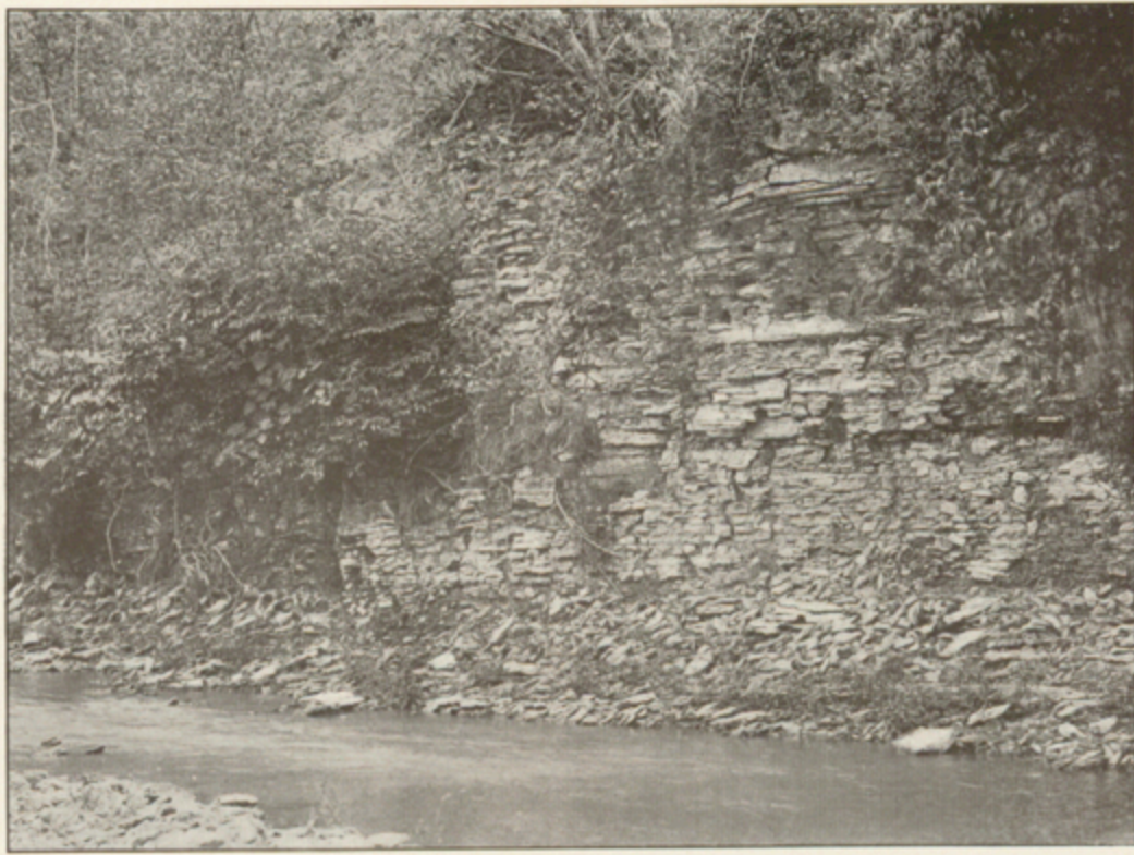
PLATE I.—LOWERMOST THIN-BEDDED PART OF GALENA DOLOMITE AT BRIDGE OVER SINSINAWA RIVER, WEST OF GALENA ILL.
