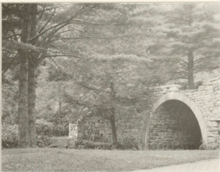
PLATE 18.—STREAM CULVERT BUILT OF WEVERTON SANDSTONE ON ABANDONED TAPEWORM RAILROAD ON FLANK OF JACKS MOUNTAIN Overgrown with large white pines
