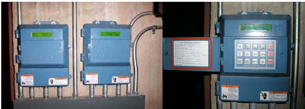
Figure 11: Magnetic Water Flow Meter in Basement of Architecture Building A
