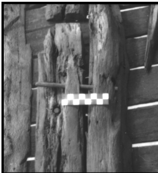
Figure 38: Drift bolt driven at a downward angle. Photo by Christopher R. Sabick.
