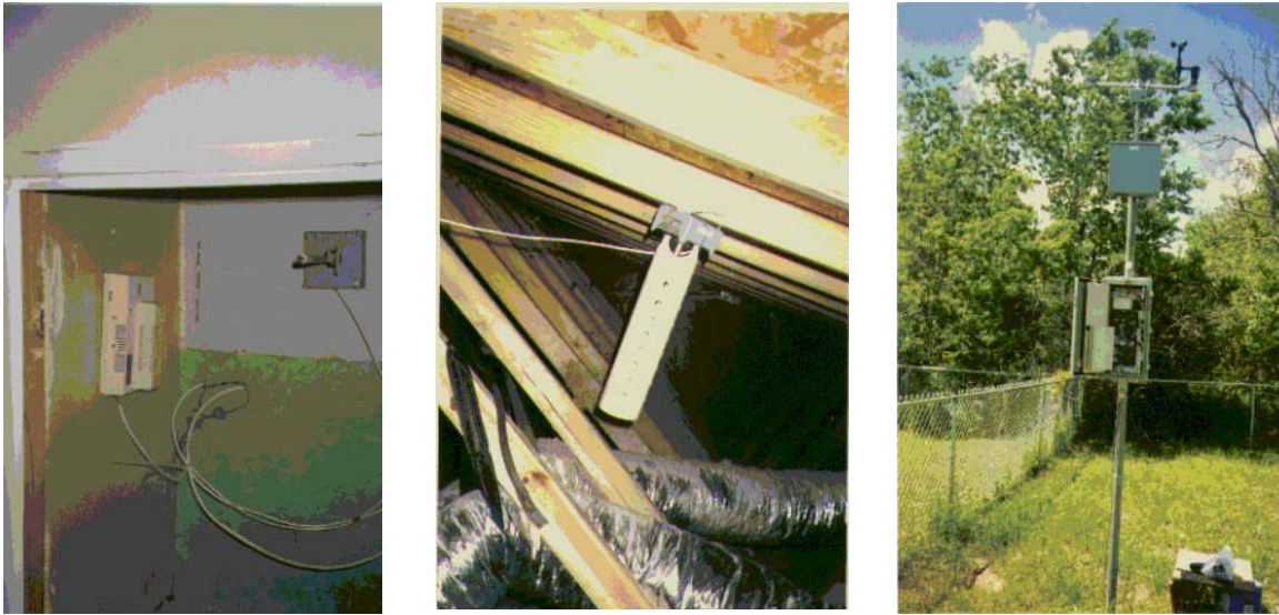
Figure 60: Sensors used in case-study house.
