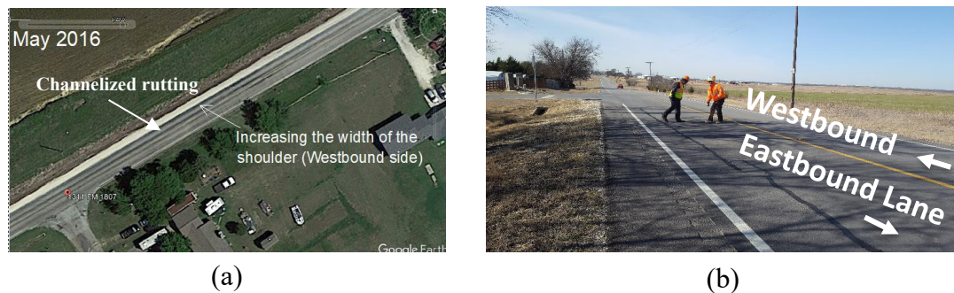
Figure 12 Pavement distresses on FM 1807: a) channelized rutting observed during May 2016, b) longitudinal cracks observed after six months of the major rehabilitation work, during January 2018
