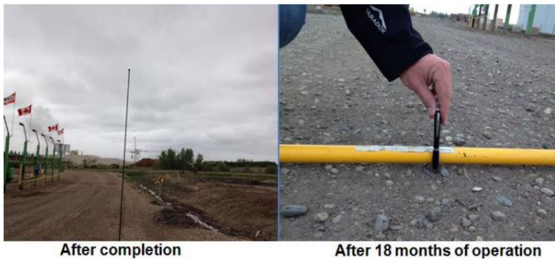
Figure 5: Condition of access road at CANFOR, Canada (Pokharel et al. 2015)
