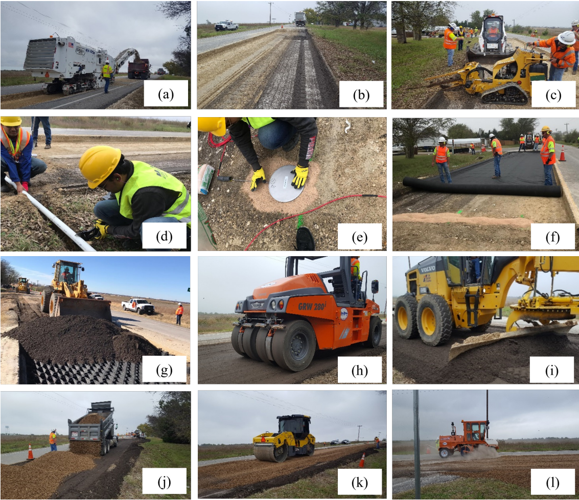
Figure 20 Construction of reinforced section 1 (RS1) with a single layer of 4-inch geocell
