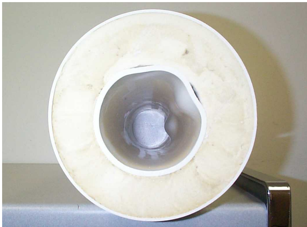
Figure 4. Inside of the PVC pipe cut from places closed to the failed sections.
