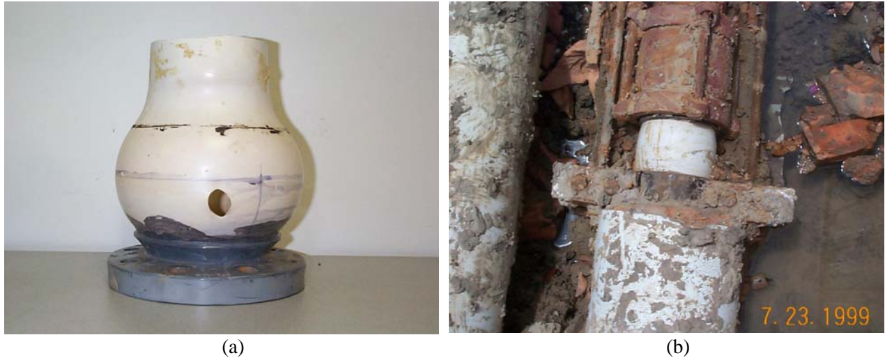
Figure 3. Failed section of the PVC pipe with flange in one end.
