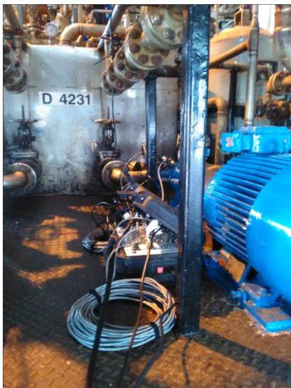
Figure 14: LO Pump A transducers connected to seismic "power box".
