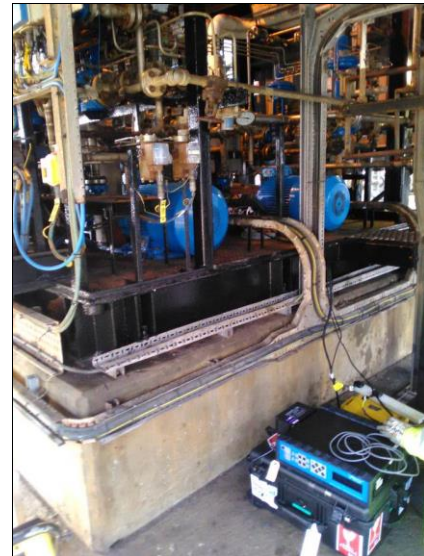
Figure 15: LO Pump A / B skid with transducers connected to DSPI.
