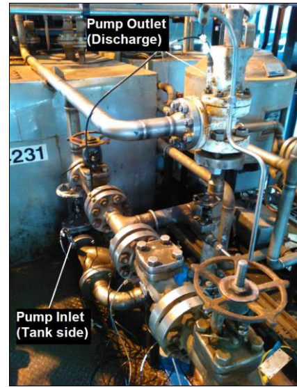
Figure 11: LO Pump A pipework with transducers fitted.
