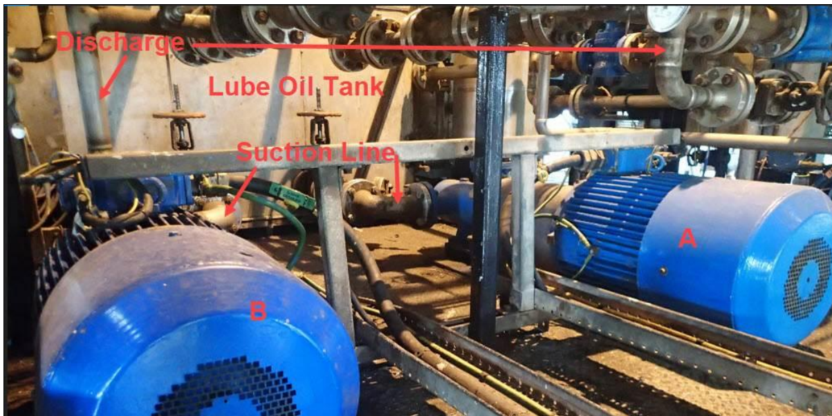
Figure 9: TEC & LO Pump A/B Skid, LO Pump side with process pipework marked up.
