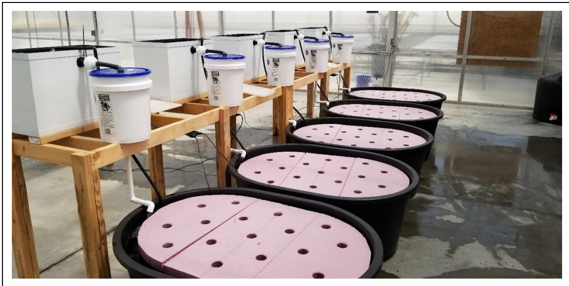
Figure 1: The floating raft hydroponic system during initial setup and plumbing leak test
