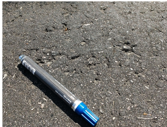
Figure 29. Surface Texture Possibly Indicating Segregation and High Air Voids.
