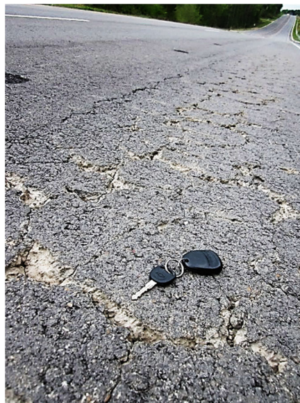
Figure 34. Premature Wheel Path Fatigue Cracking in the Outside Lane.
