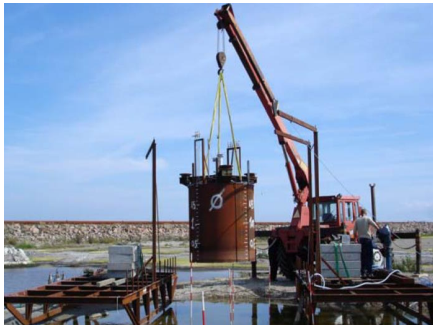
Figure 5.9: The 2 m diameter bucket used for large-scale test in Frederikshavn. Reprinted from [Houlsby et al., 2005]
