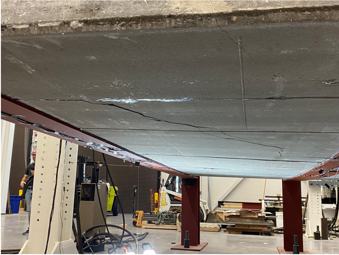
Figure 5.51: Precast panel cracking (Photo by Sheyenne Davis)
