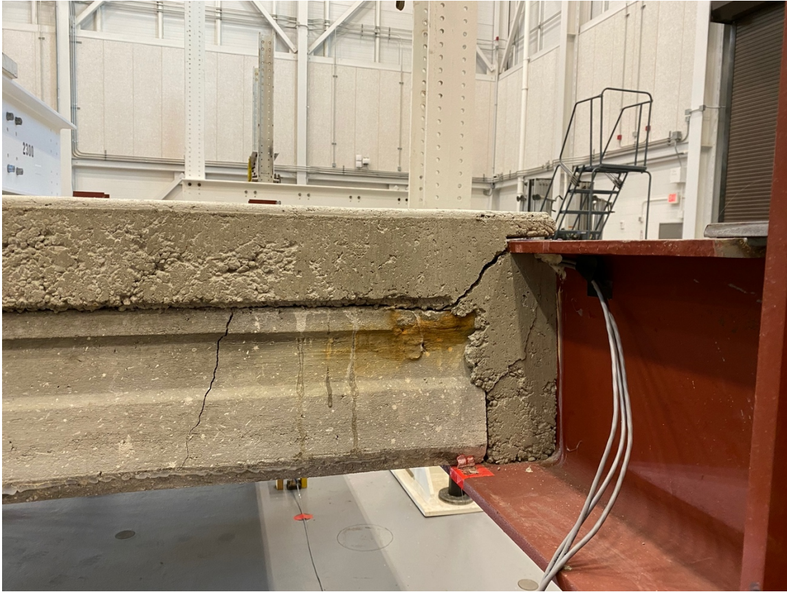
Figure 5.50: Concrete deck cracking and separation from steel beam (Photo by Sheyenne Davis)
