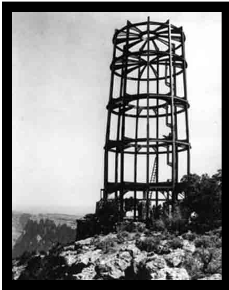
Image 17 Desert Watchtower under construction. Image courtesy of the Grand Canyon Museum Collection
