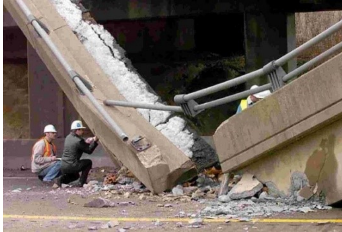
Figure 2.4: Failure of the Lake View Drive Bridge, reprinted from (Donaldson, 2005) with permission.
