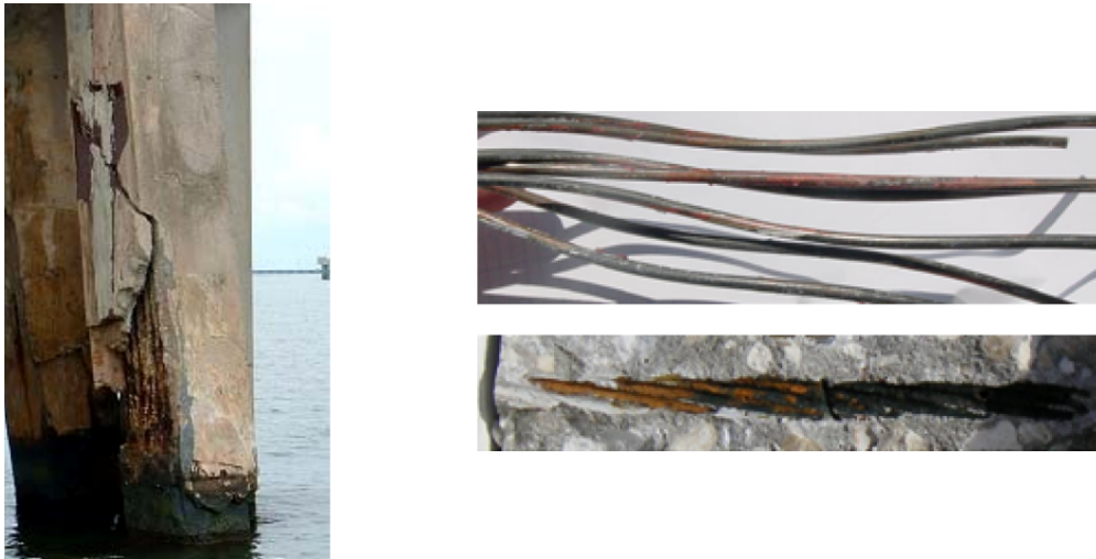
Figure 2.5: Corroded high-strength steel from the pile of the St. George Island Bridge, reprinted from (Cannon et al., 2006) with permission.
