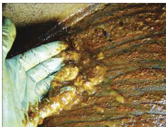
Figure 4: Sludge formed from lubricating oil. Reprinted from Livingstone et al. (2007).
