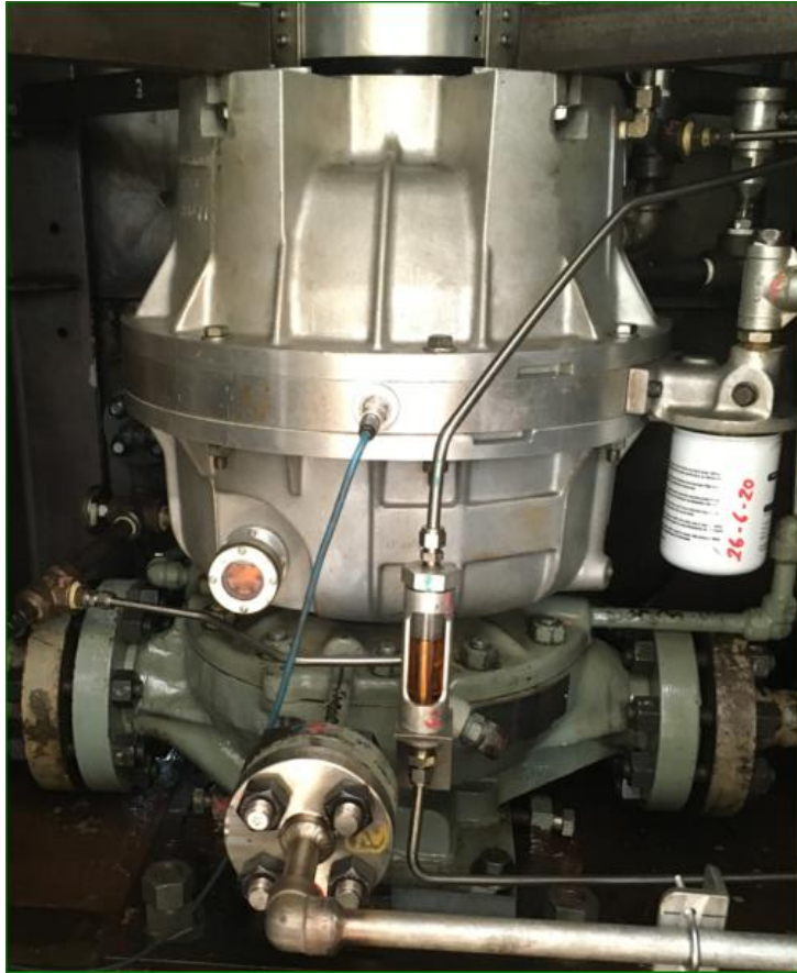
Figure: Pump at site
