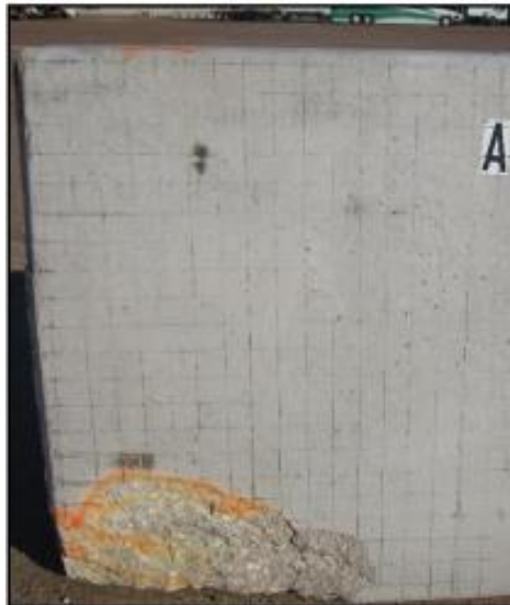
Figure 22. Region 4 towards the end of Barrier A. Part of the base at the left end has a spall with no exposed reinforcement.
