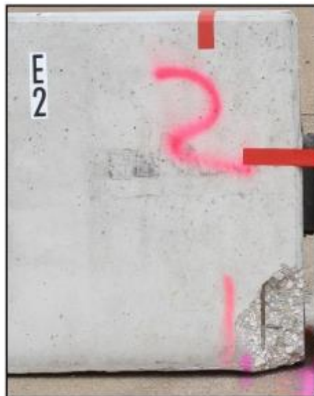
Figure 54. Barrier which is Acceptable with Repair—Spalled Region Where Reinforcement May Have Some Exposure but Does Not Protrude
