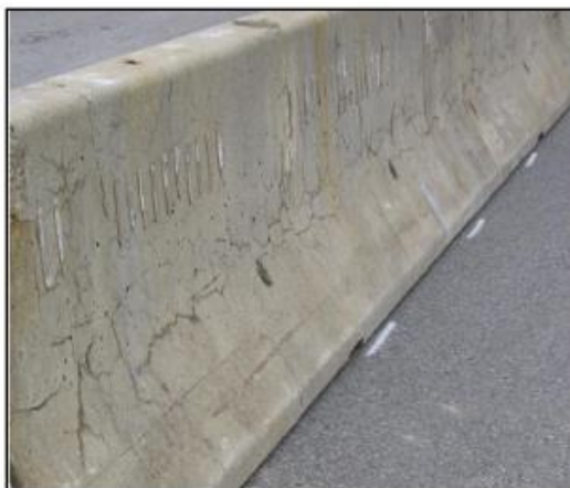
Figure 67. Acceptable Barrier—Compressed Longitudinal Crack in the Lower Half of the Barrier Stem (Bottom 50 Percent of the Total Height) (2). Reprinted from Temporary Barrier Guidelines-Longitudinal Cracks, NYSDOT.
