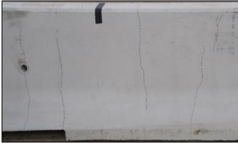
Figure 64. Compressed Transverse Cracks: A Decision May Not Be Made Immediately.
