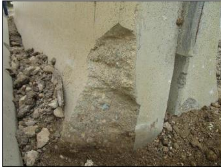
Figure 57. Unacceptable Barrier—Spalled Dimension Equal to 12 Inches and Spall Depth Less than the Cover; Reinforcement Is Not Exposed.
