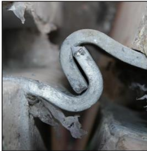
Figure 71. Unacceptable Barrier—Rotated JJ Hooks Coming from Different Ends; The Ability of This Connection to Redirect an Errant Vehicle Will Be Reduced.
