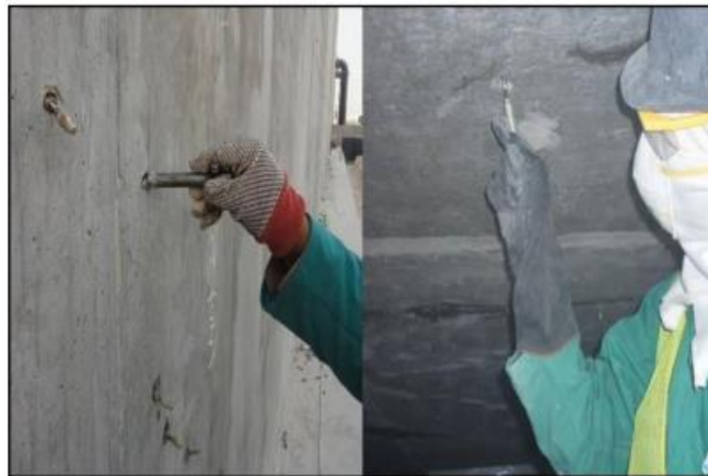
Figure 78. Installing Injection Ports (6). Reprinted from “Concrete Repairing by Epoxy Injection”, Design Consulting Services.
