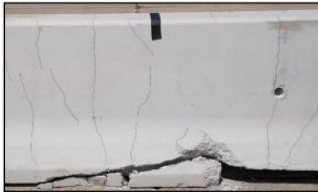
Figure 70. Unacceptable Barrier—Missing Section near the Edge of the Scupper.
