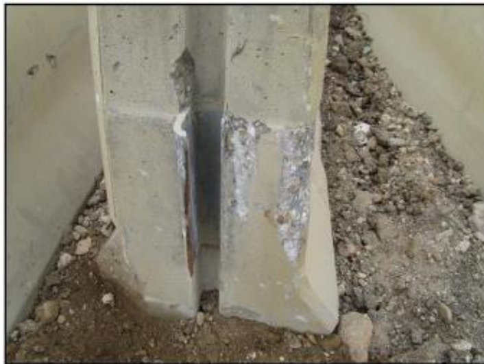
Figure 73. Unacceptable Barrier—JJ Hook Failure by Brittle Fracture.
