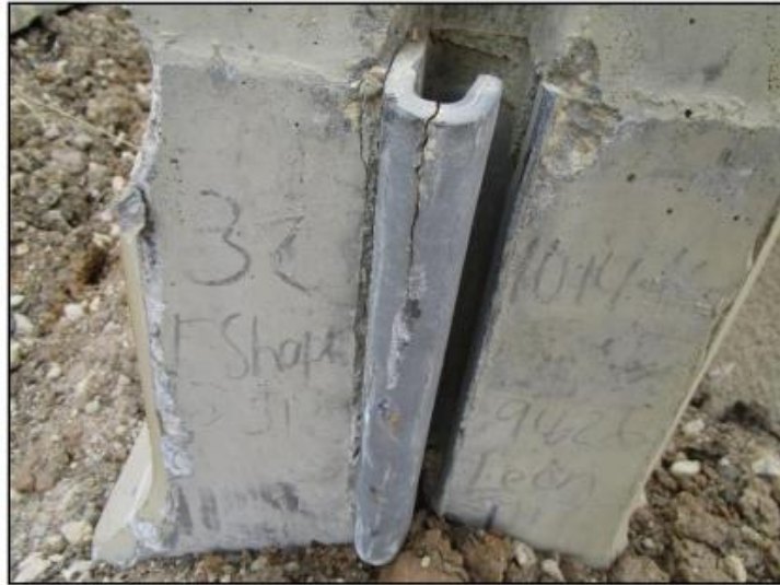
Figure 75. Unacceptable Barrier—Cracked JJ Hook.
