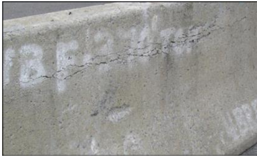
Figure 6. Clustered Horizontal Cracks due to the Tight Clamping of Lifting Devices (10). Reprinted from Temporary Barrier Guidelines-Longitudinal Cracks, NYSDOT.
