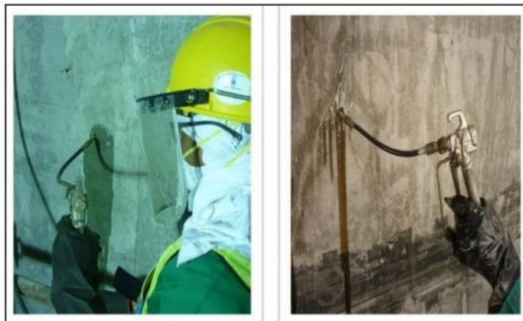
Figure 79. Injection of Epoxy Resin into the Holes (6). Reprinted from “Concrete Repairing by Epoxy Injection”, Design Consulting Services.
