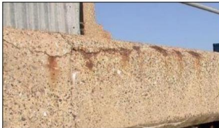
Figure 11. Crack due to the Corrosion of Reinforcement (24). Reprinted from concrete.org.uk
