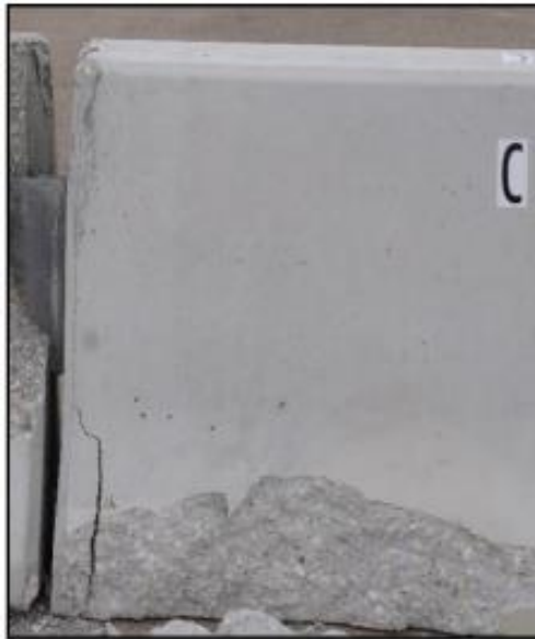
Figure 55. Unacceptable Barrier—Large Chunk of Partially Broken Concrete Piece from the Toe Susceptible to Break Off When Further Impacted.
