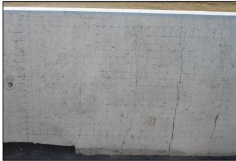
Figure 19. Region 1 with transverse cracks gradually increasing in width (left to right), Barrier E.
