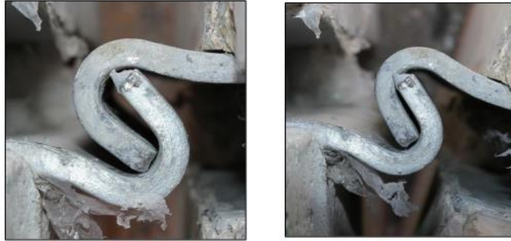
Figure 15. Stages of deformation of the joint between the single slope barriers E and A.
