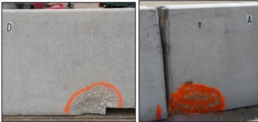
Figure 60. Unacceptable Barrier—Spall Projects towards Traffic by More than 30 Degrees.
