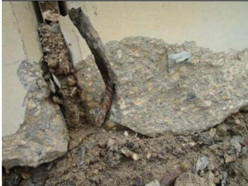
Figure 3. Corrosion of Reinforcing Bar Embedded in the Toe of the Concrete Barrier.
