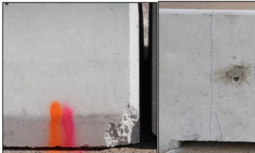
Figure 58. Acceptable Barrier— Spalled Dimension Less than 12 Inches and Spall Depth Less than the Cover; Reinforcement Is Not Exposed.
