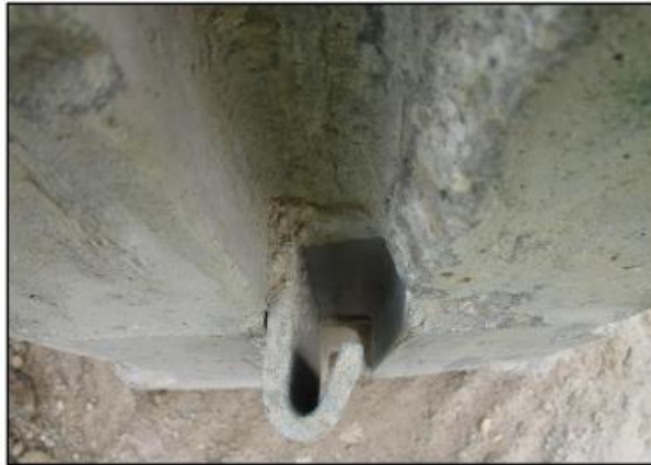
Figure 72. Unacceptable Barrier—Rotated JJ Hook at the End; a Connection Will Be Difficult to Form.
