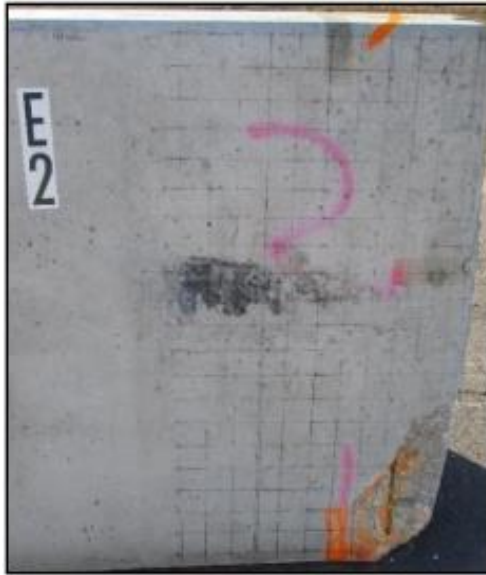
Figure 20. Region 2 at the extreme end of Barrier E. Right corner has a spall with exposed reinforcement.
