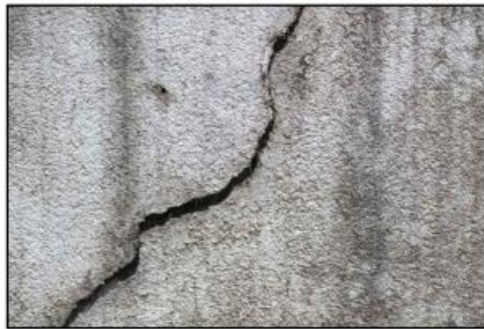
Figure 10. Crack due to the Formation of More Voluminous Products (22). Reprinted from gharpedia.com
