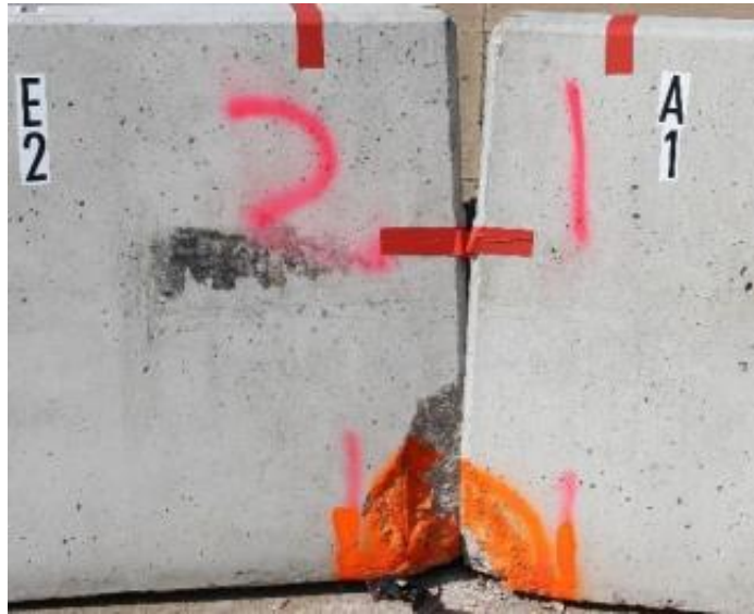
Figure 4. Spalling at the Toe of Barrier E due to a Vehicle Crashing into the Joint between Barriers A and E.
