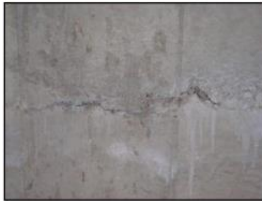
Figure 12. Crack-Like Formation due to the Lack of Mixing of Two Batches of Concrete during the Pour (21). Reprinted from waterstopsolutions.com
