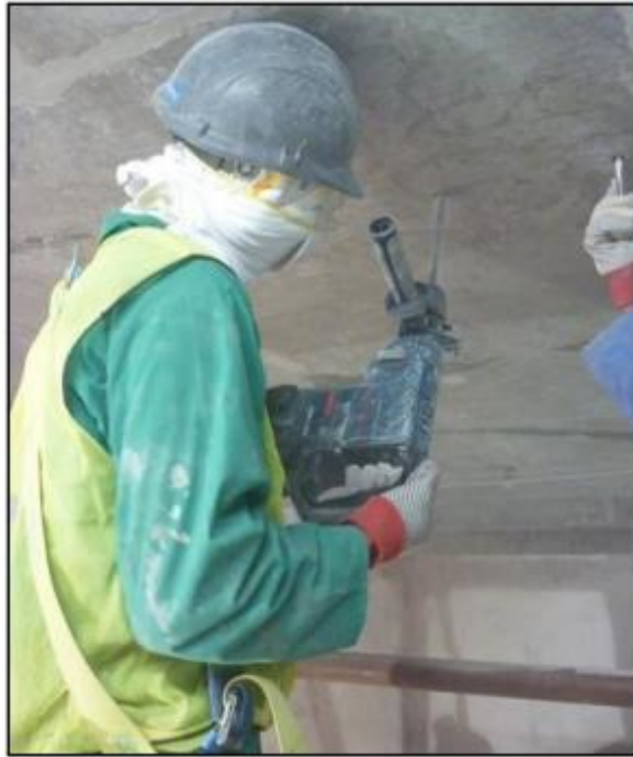
Figure 76. Drilling Holes in the Concrete Member (6). Reprinted from “Concrete Repairing by Epoxy Injection”, Design Consulting Services.
