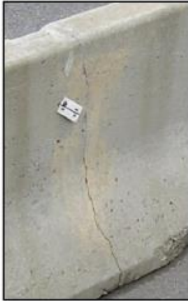
Figure 69. Barrier which is Acceptable with Repair—Single Transverse Crack with No Evidence of Corrosion (3). Reprinted from Temporary Barrier Guidelines-Cracked Sections, NYSDOT.
