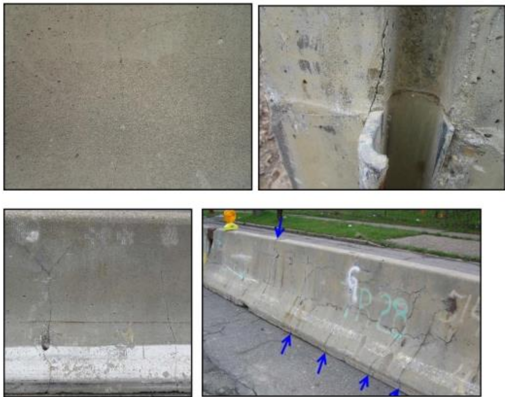
Figure 5. Cracking in Portable Concrete Barriers (8). Reprinted from Temporary Barrier Guidelines-Cracked Sections, NYSDOT.
