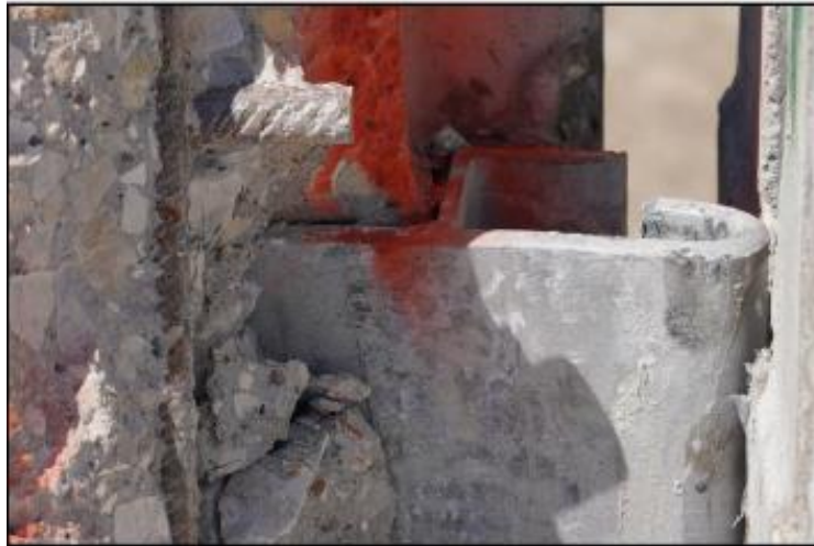
Figure 53. Unacceptable Barrier—Spalling beyond the Outer Layer of Rebar Embedded within the Barrier, Exposing It and Making It Protrude.
