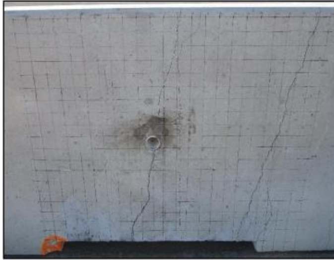
Figure 21. Region 3 on Barrier A, encompassing cracks gradually increasing in their width.
