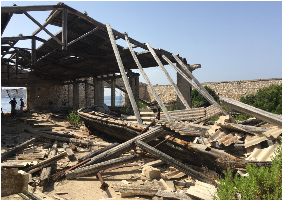
Figure 16: The collapse of the shed roof on the Isola di Capo Passero meant disaster for the several mattanza boats under its shelter. Image by the author, 2019. © Claire Zak 2019.
