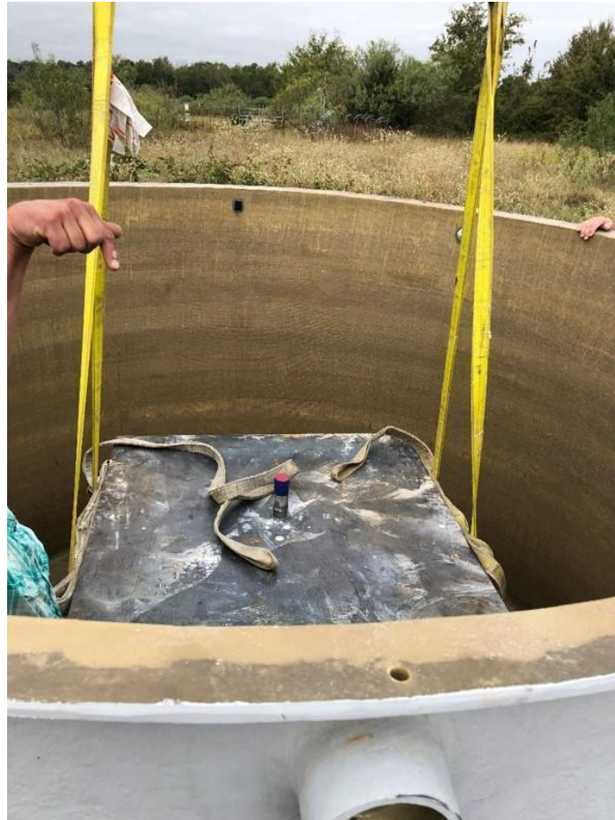
Figure 15. Block and tank setup
