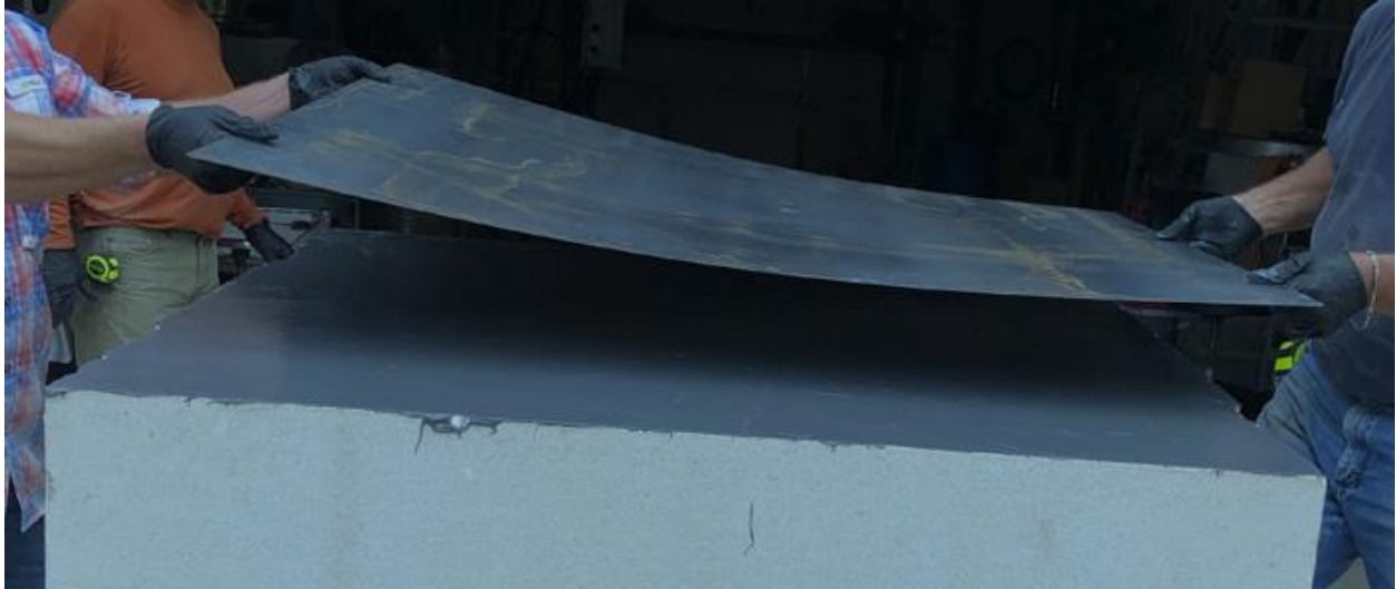
Figure 7. Bottom steel plate and epoxy layer
