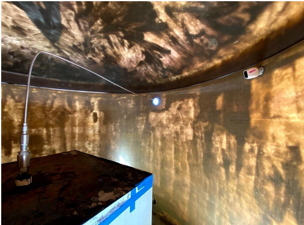
Figure 27. Arlo camera mounted in tank
