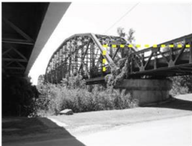
The Colorado River Bridge is a 2-part, steel truss and concrete highway bridge crossing the Colorado River on a north-south axis, Pennsylvania through truss bridge over Colorado River on Business 59 SB in Wharton Built 1930.
