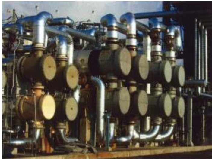
Figure 4. Bank of heat exchangers in refinery – Courtesy The Process Technology and Operator Academy
