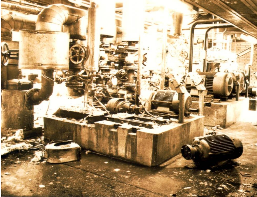
Figure 4: Damage caused by a running blocked-in water pump
