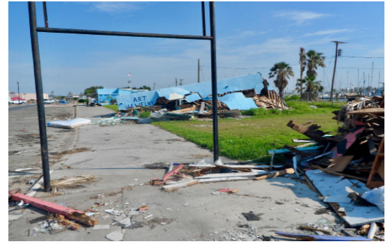
Figure 8.16: Hurricane Harvey's destruction of the Heritage District Picture Courtesy: Kate de Gennaro
