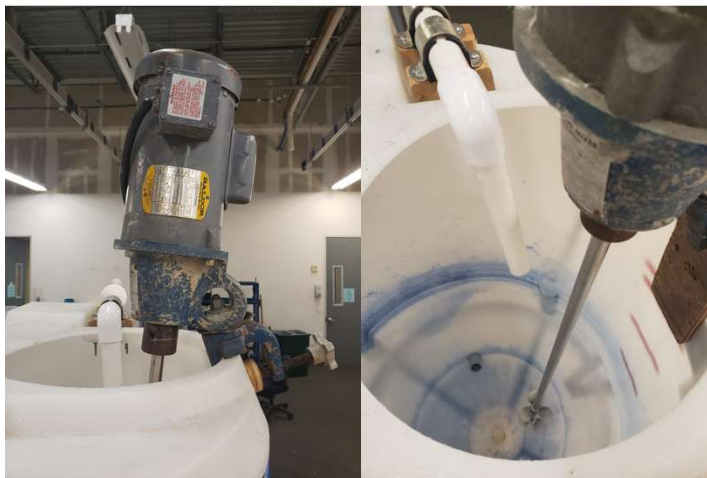
Figure 16. Mixing motor with two propellers installed on bottom to agitate fluids.
