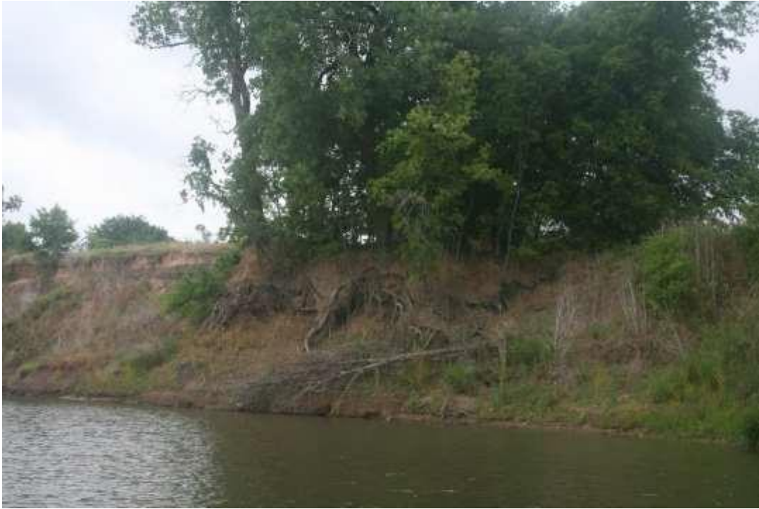
Figure 154: The western bank experiences increased erosion as it grades to a cutbank.
