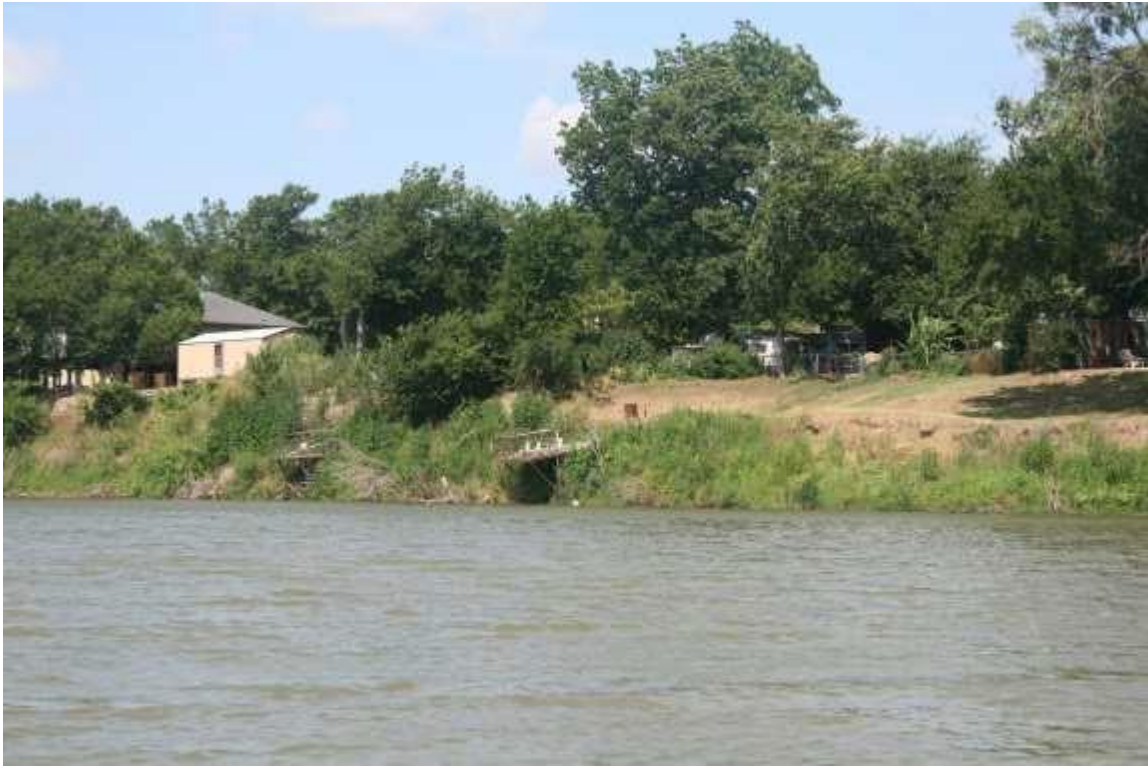
Figure 169: Note that the dock on the right is leaning into the river channel.
