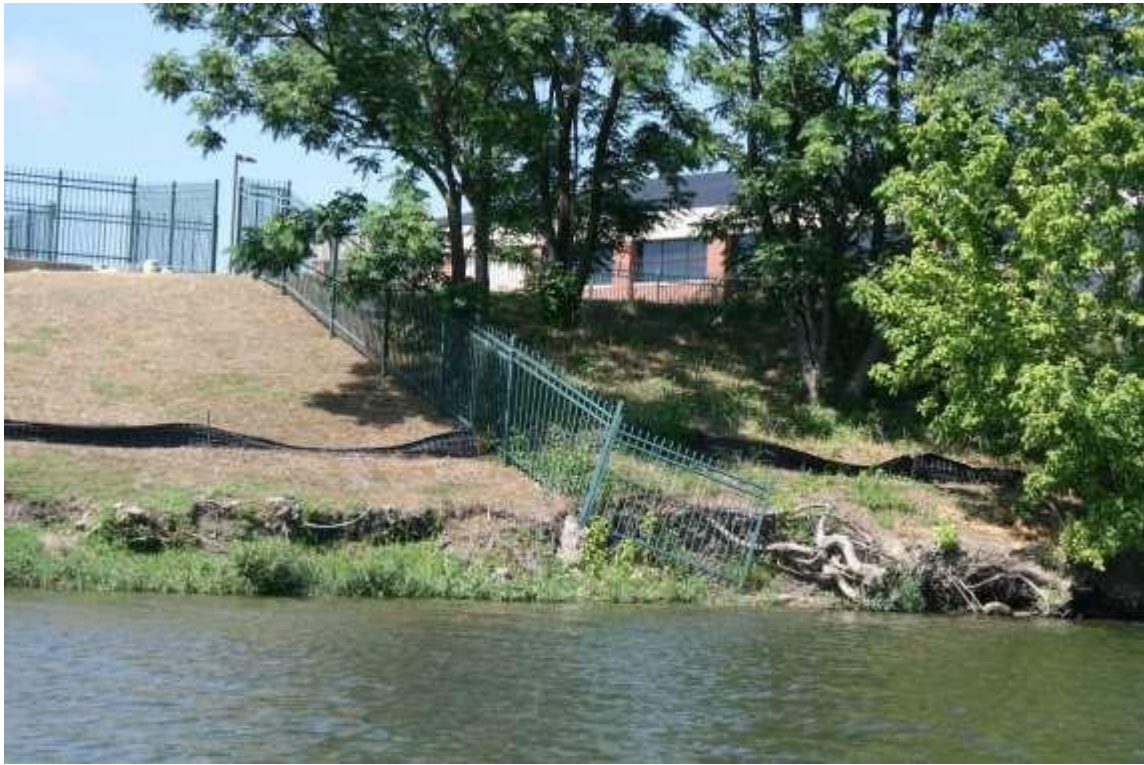
Figure 143: Fence failure resulting from bank slump
