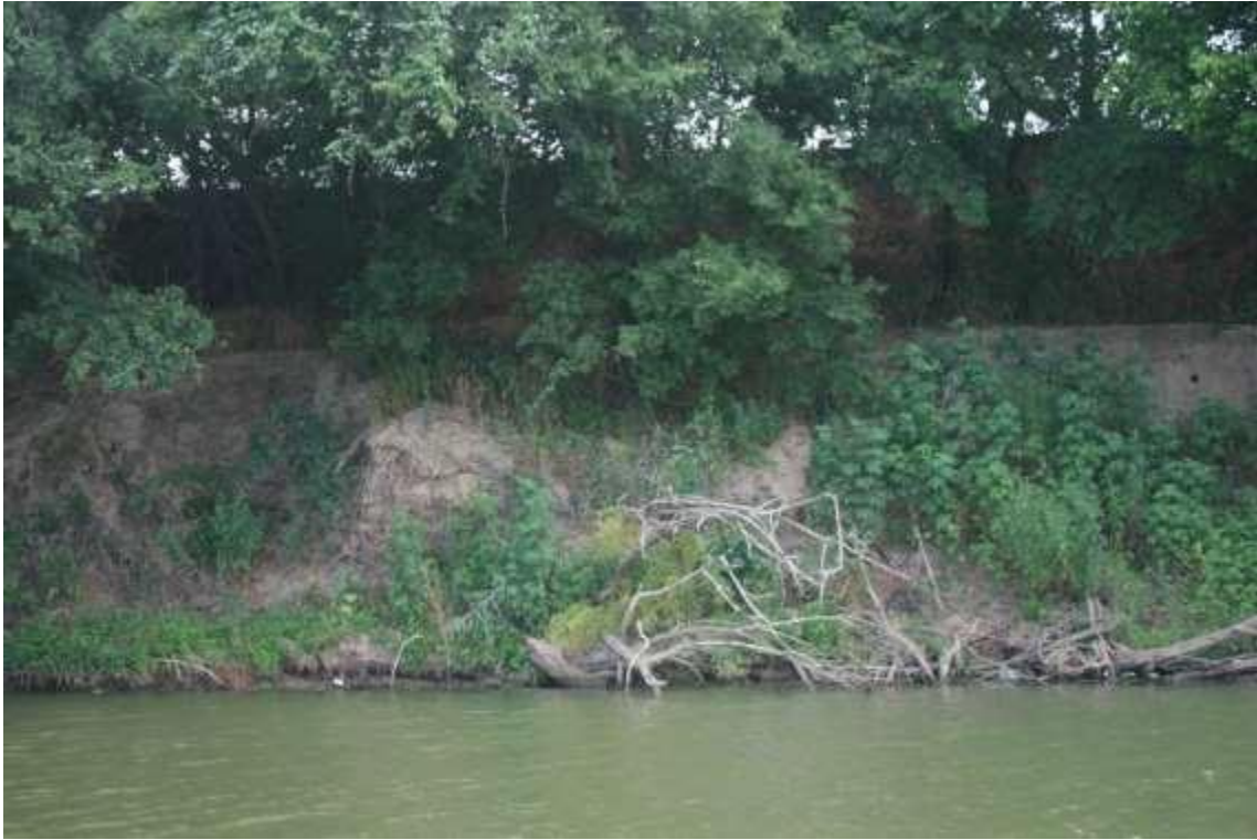
Figure 159: Bank cutting and erosion was extensive at BR20.
