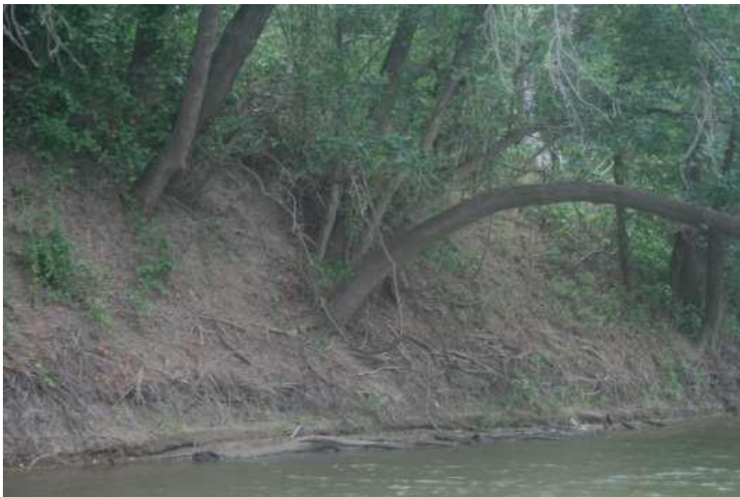
Figure 149: Bank cutting and exposed roots at BR17.
