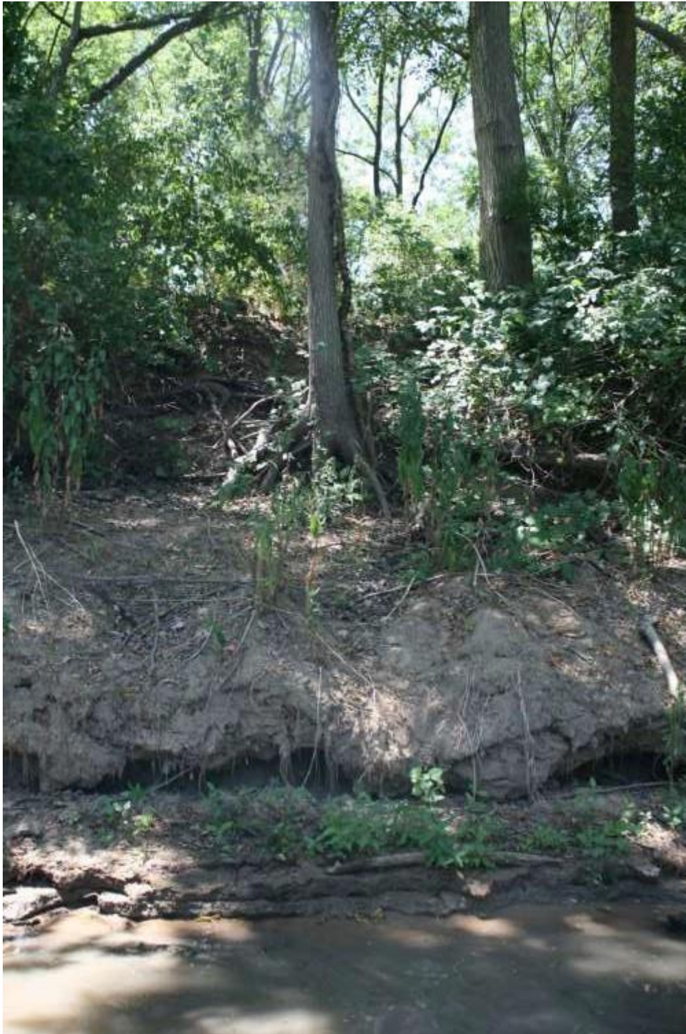
Figure 115: One of the more severe cuts at BR07.
