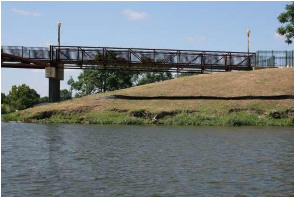
Figure 142: On southern bank, bank erosion is extensive.
