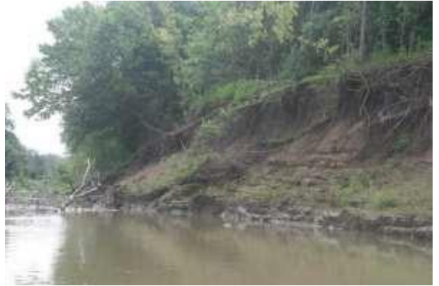
Other sections had increased channel erosion with exposed roots.
