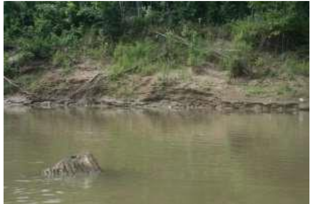
Small slump near Location 5.
