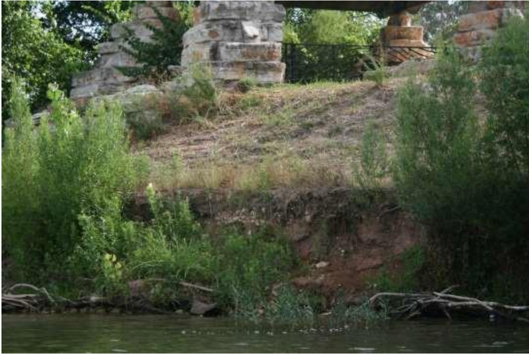
Figure 129: Localized bank instability is seen immediately adjacent to engineering structures.
