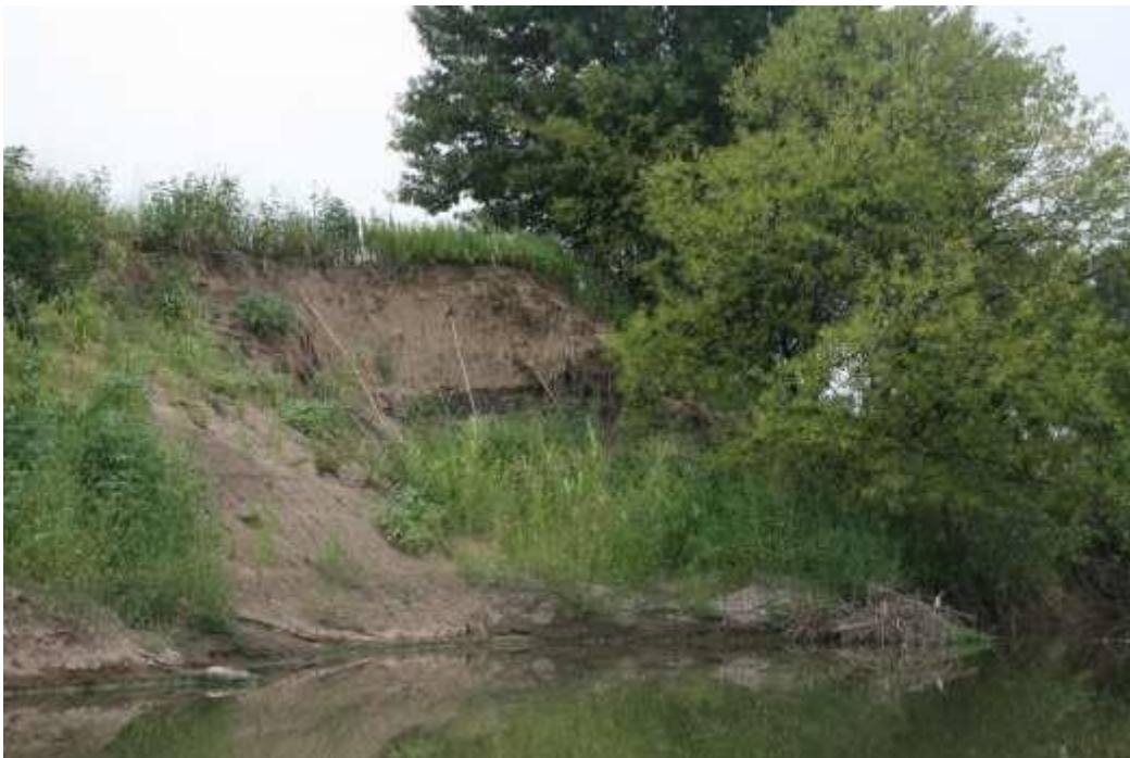
Figure 180: Cutting and bank failure at TR01. Cutting was not continuous, but serious where present.
