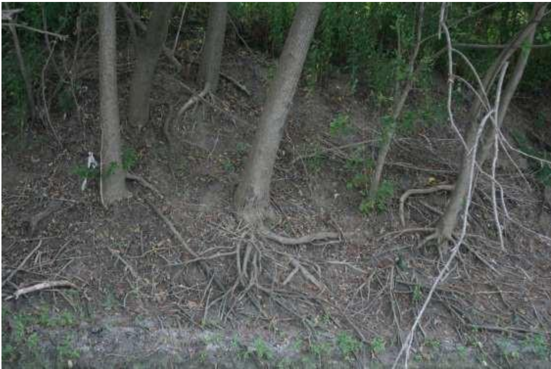
Figure 162: Exposed roots at BR21
