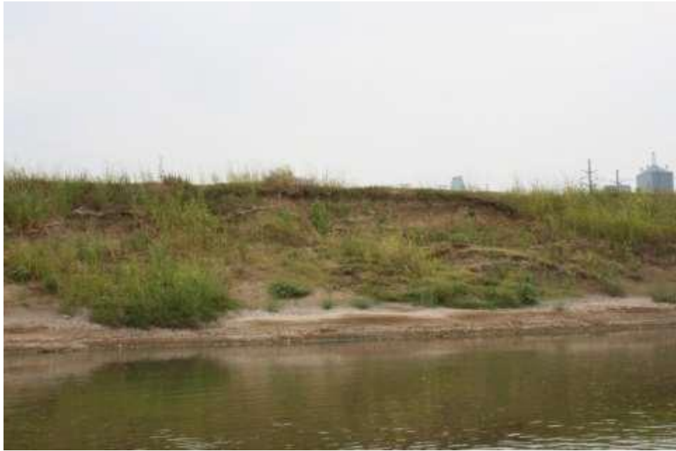
Figure 193: Slump on northern bank at TR06
