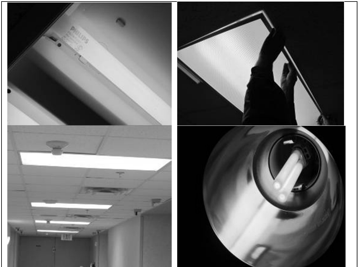
Figure 3.12. Electric lighting at facility three.
