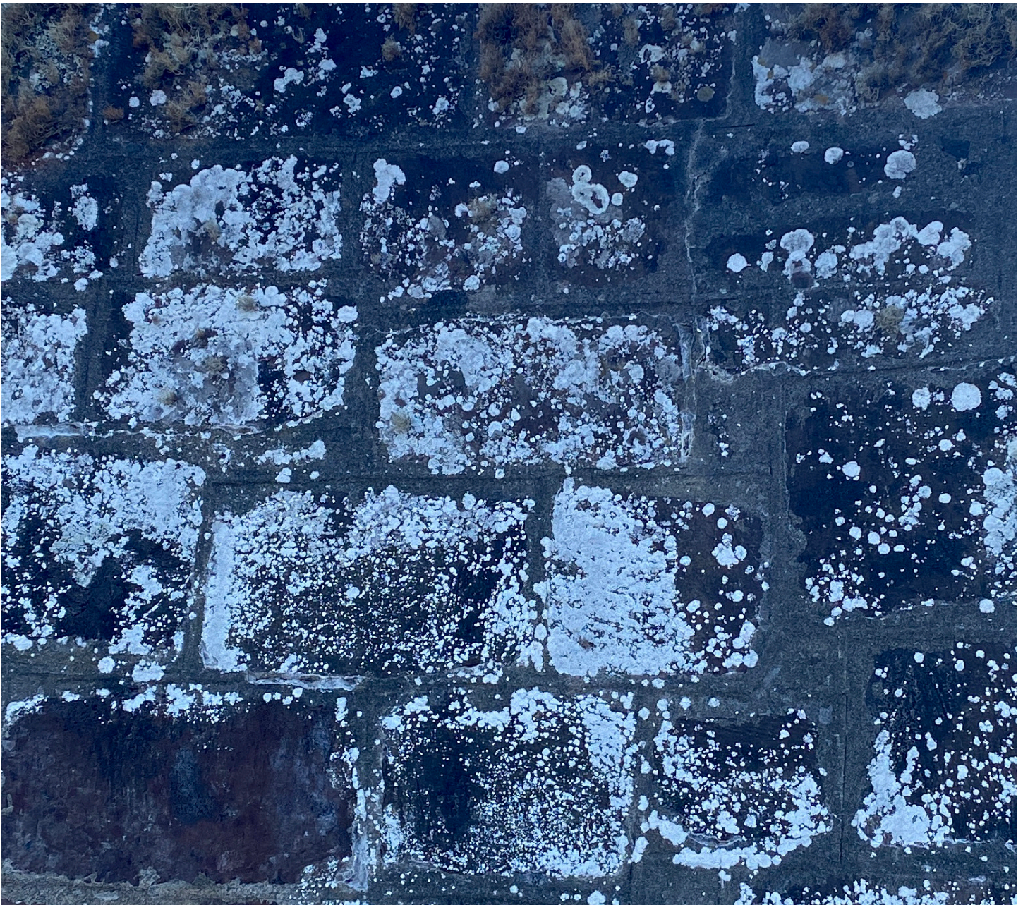
Figure 58: Efflorescence detail on the firing platform of the southern complex (Image: B. Fortenberry).
