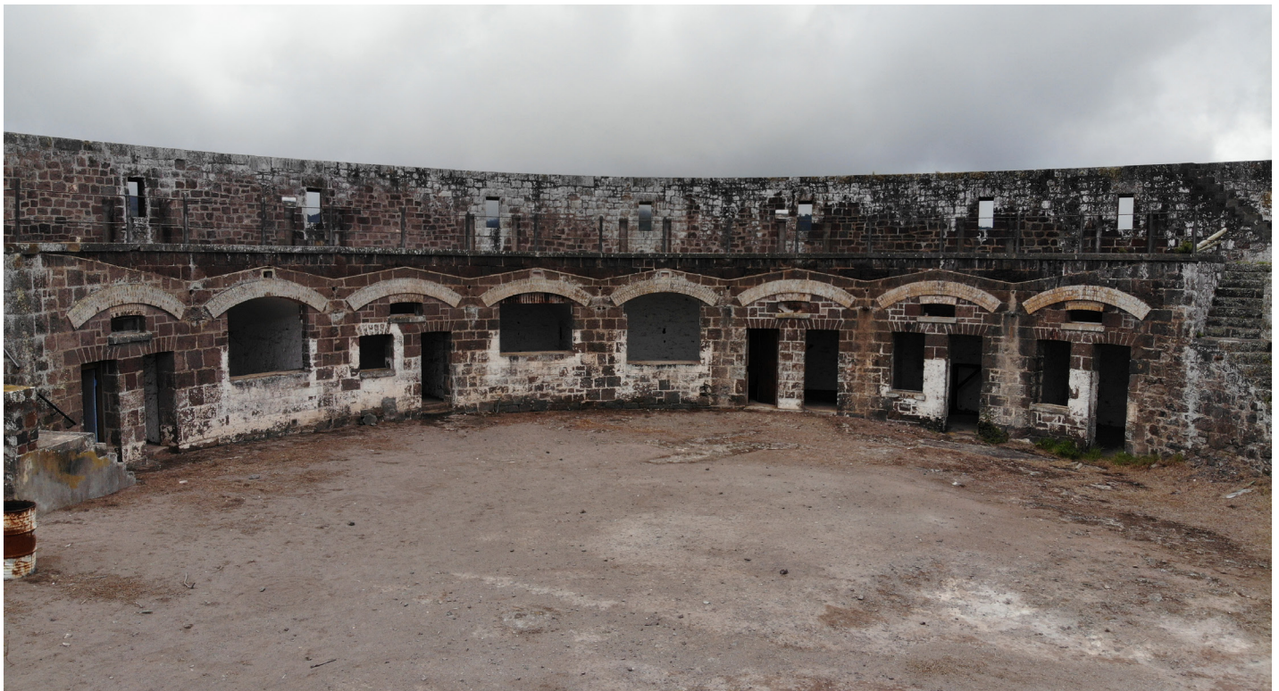
Figure 60: Efflorescence on the northern face of the southern firing platform (Image: B. Fortenberry).
