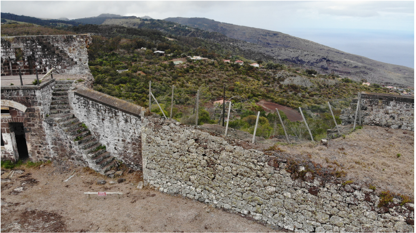
Figure 65: Danger sign and failing fencing near southwestern wall collapse (Image: B. Fortenberry).
