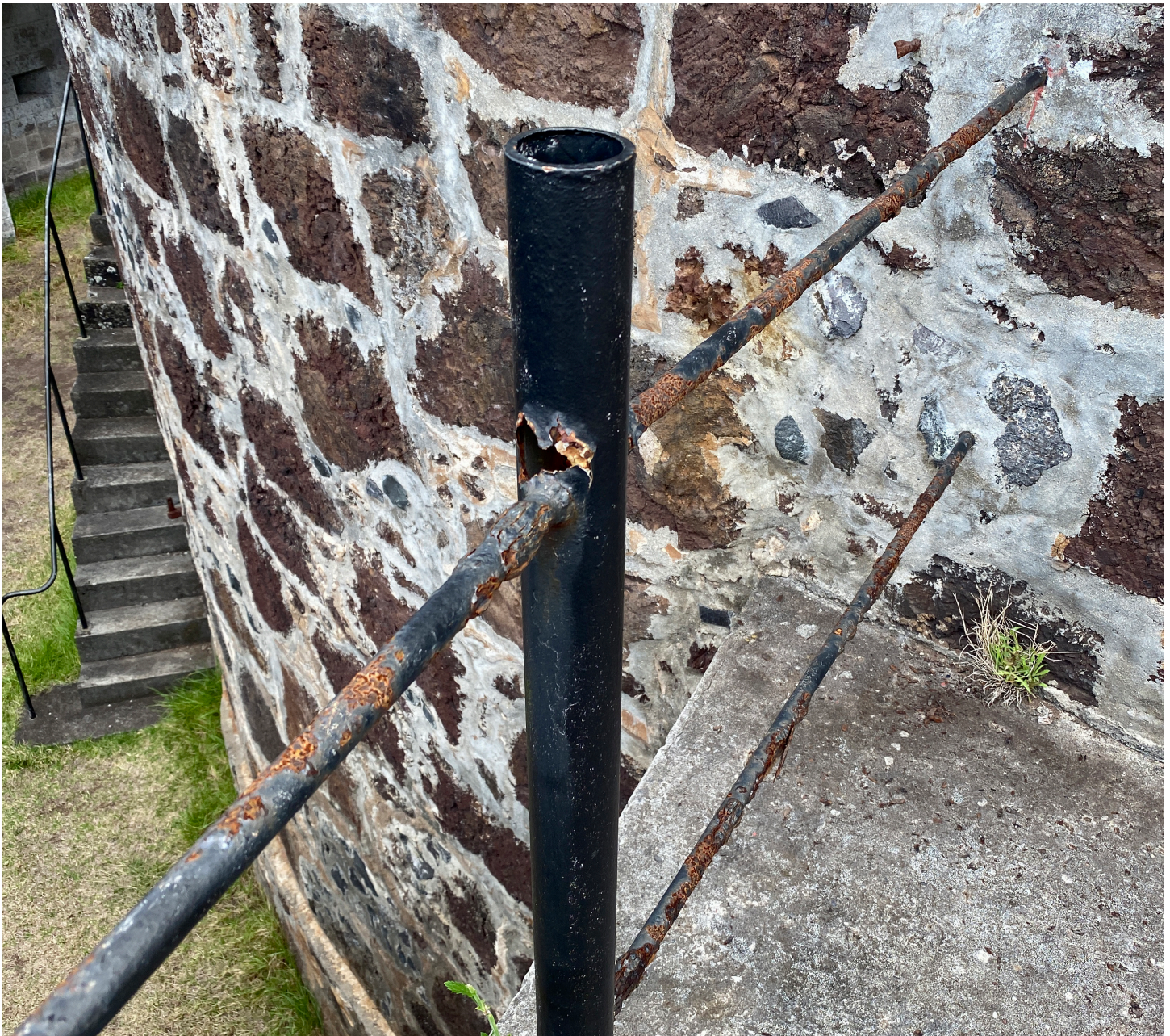
Figure 61: Cast iron pier and guard rail failure in northern complex (Image: B. Fortenberry).
