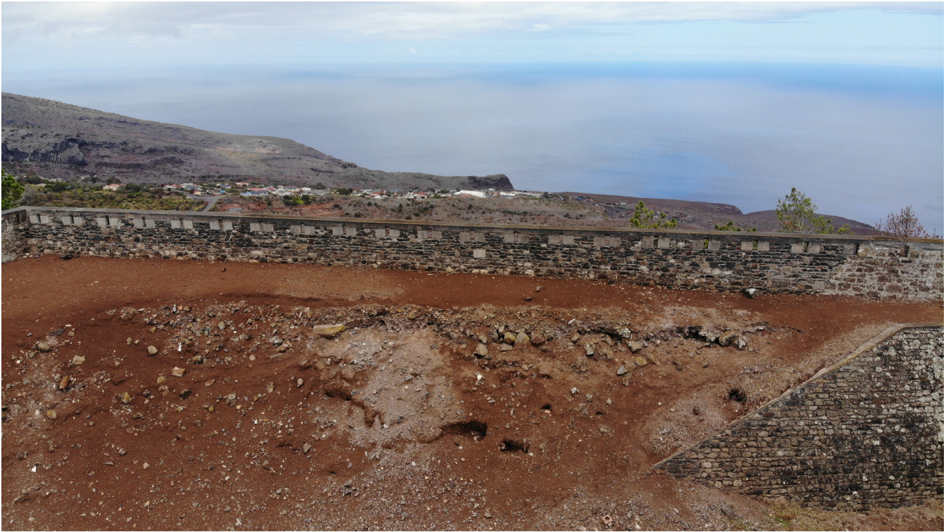
Figure 33: Aerial view of western interior wall section with erosion of 21st century infill in detail (Image: B. Fortenberry).
