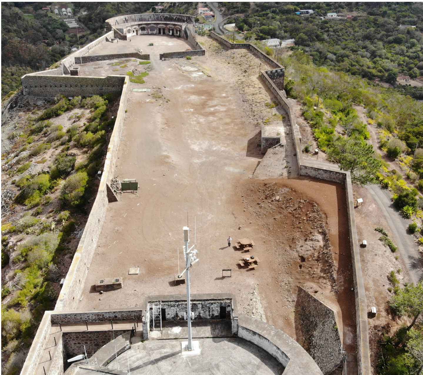
Figure 32: Aerial view of northern terminus of fort interior, erosion in detail in the right portion of image (Image: B. Fortenberry).
