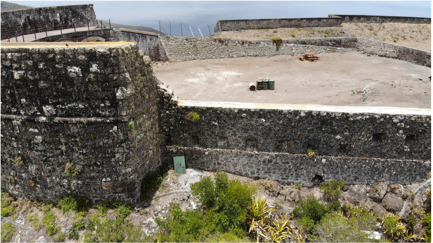
Figure 49: Aerial image of bio-growth on the eastern wall (Image: B. Fortenberry).
