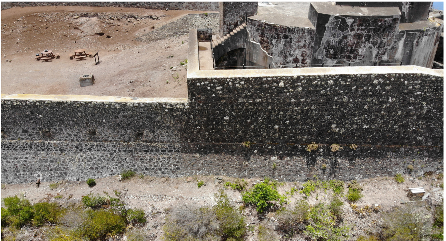
Figure 52: Aerial image of bio-growth on the northeastern wall (Image: B. Fortenberry).
