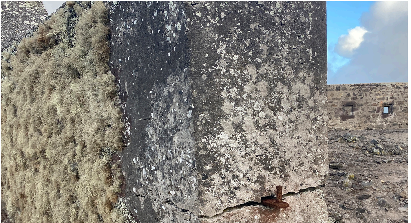
Figure 56: Detail of bio-growth on the interior fort wall (Image: B. Fortenberry).
