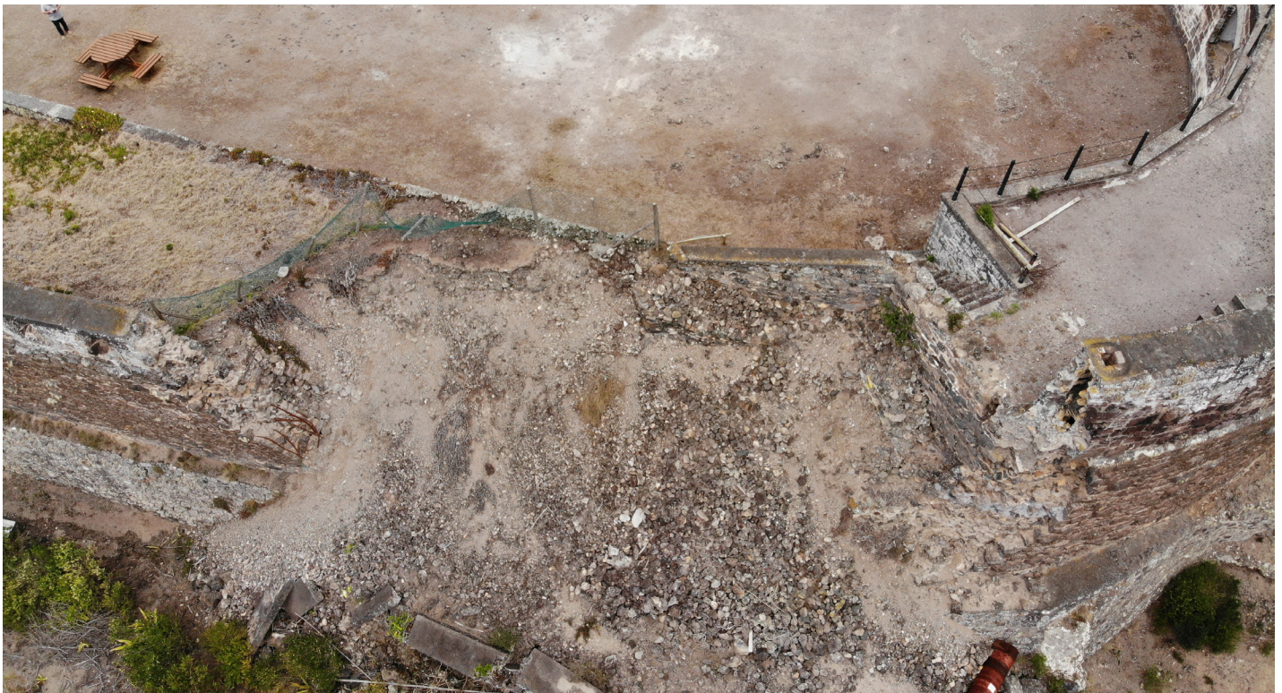
Figure 23: Nadir aerial view of wall collapse from southwest corner with top of collapse in detail (Image: B. Fortenberry).
