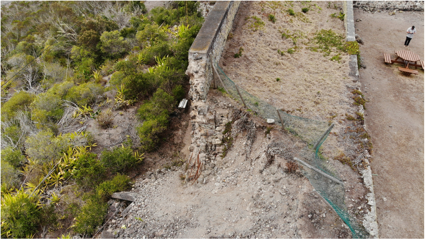
Figure 28: Aerial view of wall collapse in southwest corner looking north, western failed wall section in detail (Image: B. Fortenberry).
