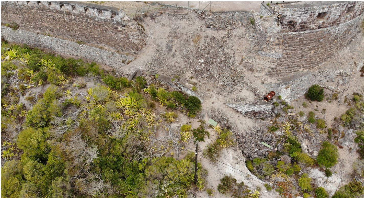
Figure 21: Nadir aerial view of wall collapse from southwest corner with base of collapse in detail (Image: B. Fortenberry).
