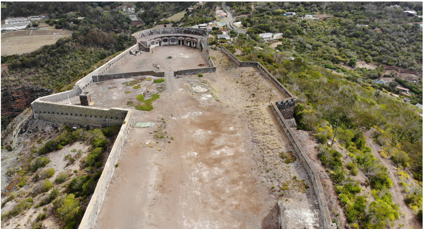
Figure 31: Aerial view of wall collapse from the northern edge of the fort complex, image looks south (Image: B. Fortenberry).
