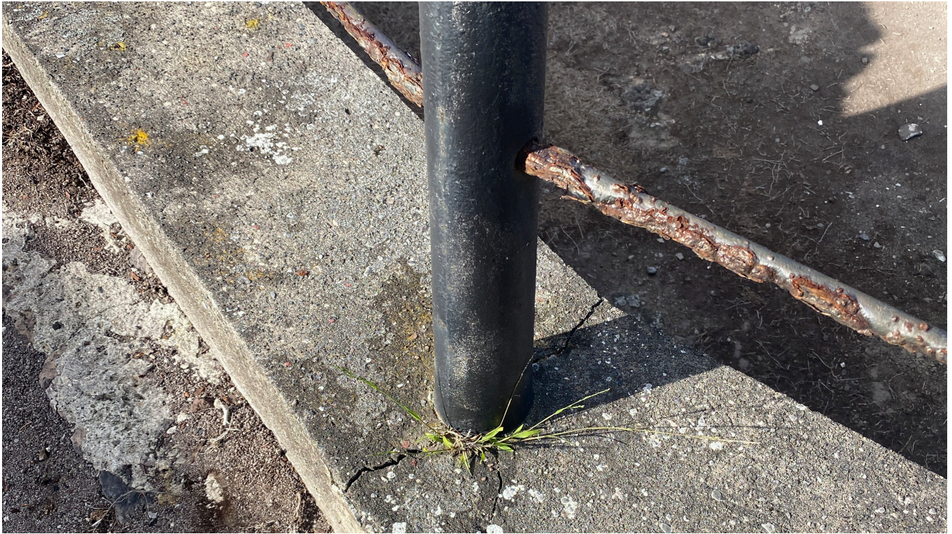
Figure 62: Cast iron pier failure and rust jacking in concrete footing on southern firing platform (Image: B. Fortenberry).
