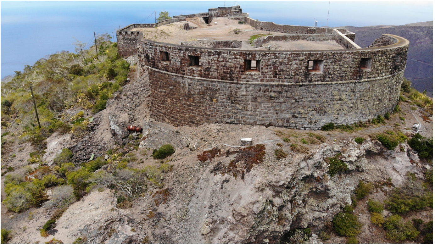
Figure 30: Aerial view of wall collapse in southwest corner from the southern exterior of the fort (Image: B. Fortenberry).
