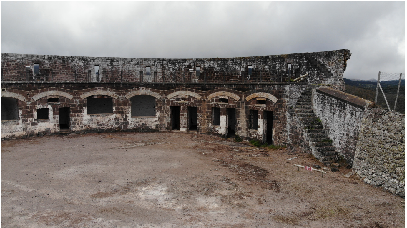
Figure 56: Soiling on the interior wall of the southern complex (Image: B. Fortenberry).
