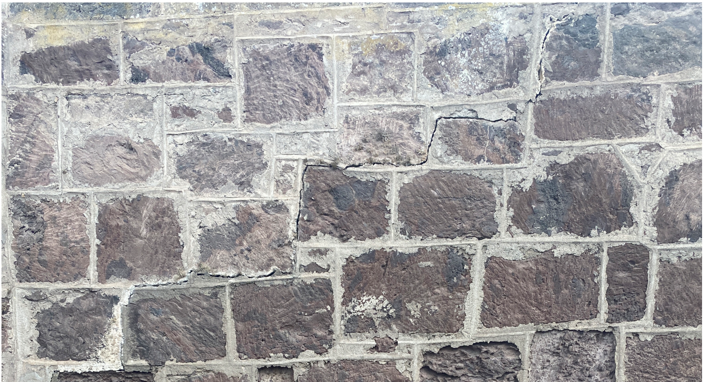
Figure 41: Detail of Portland based mortar with raised joints in detail (Image: B. Fortenberry).
