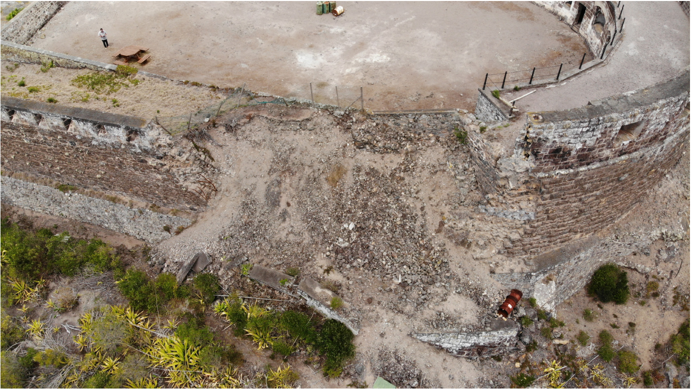
Figure 22: Nadir aerial view of wall collapse from southwest corner with base of collapse in detail (Image: B. Fortenberry).
