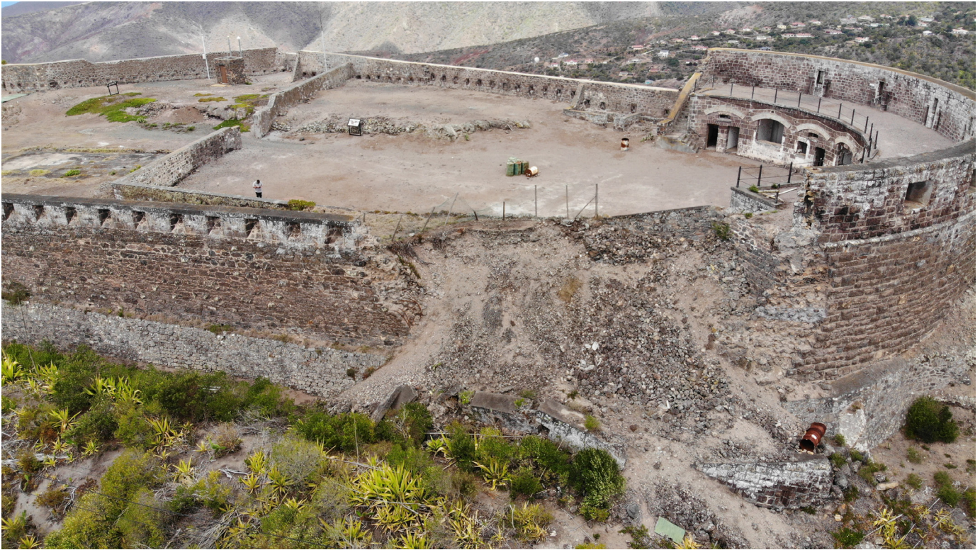
Figure 20: Oblique Aerial view of wall collapse from southwest corner of fort looking east (Image: B. Fortenberry).
