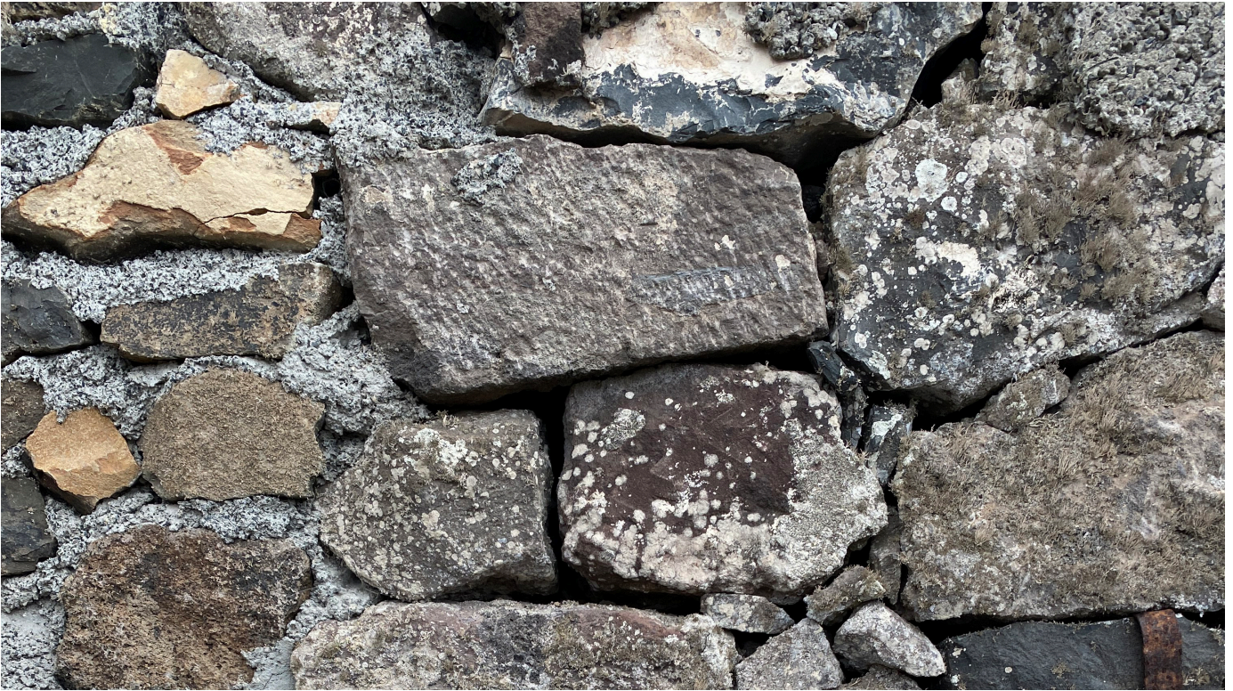
Figure 42: Detail of Portland based mortar and dry-laid stone in detail, bio-growth also present (Image: B. Fortenberry).
