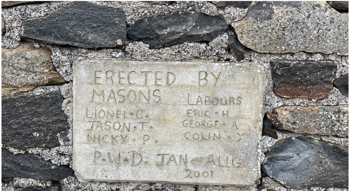
Figure 36: Detail of Portland based mortar with date plate from 2001 (Image: B. Fortenberry).
