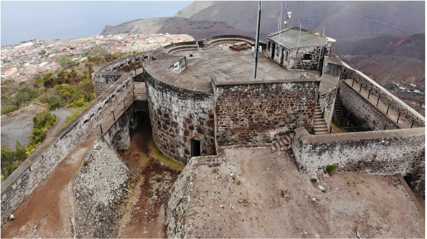
Figure 59: Efflorescence on the southern face of the northern tower complex (Image: B. Fortenberry).
