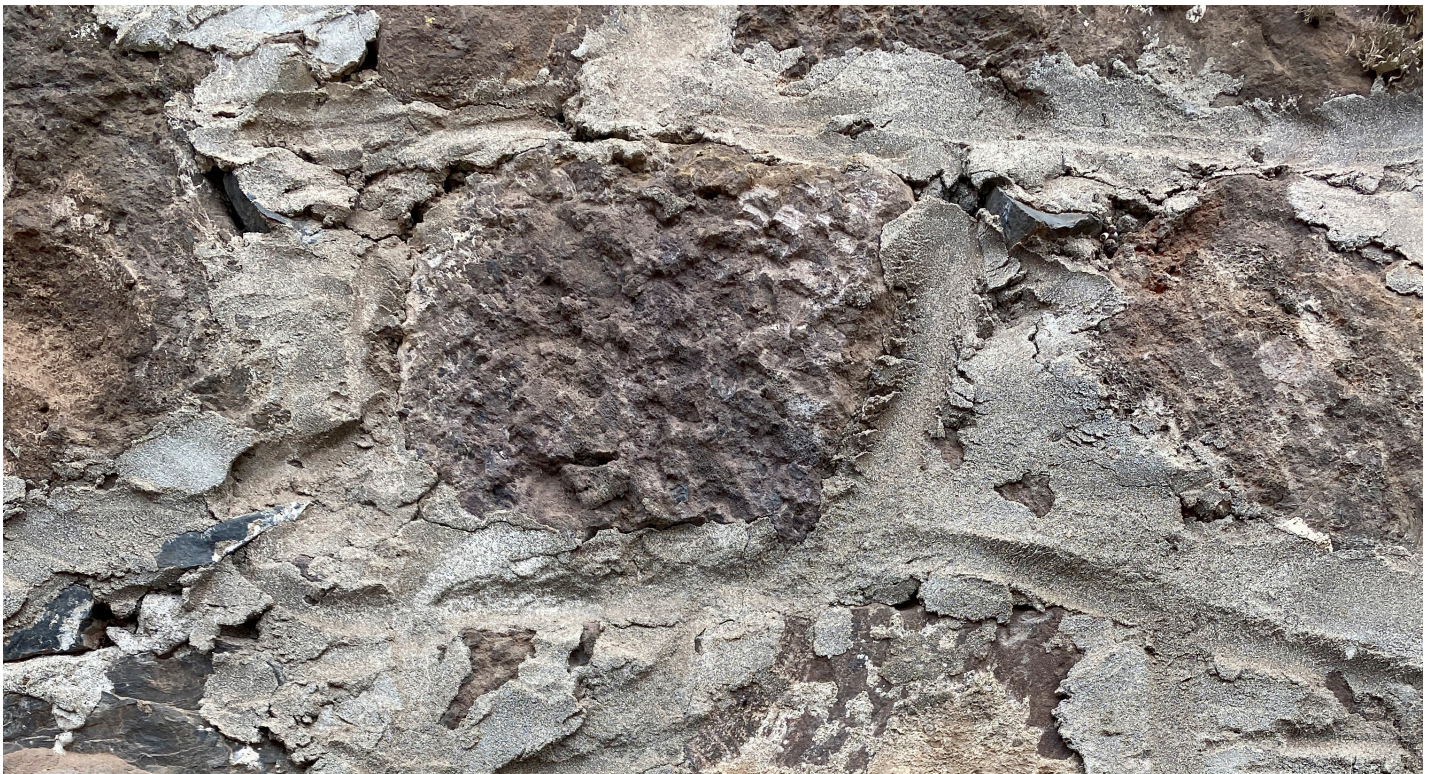
Figure 43: Detail of Portland based mortar with raised joints and haphazard application in detail (Image: B. Fortenberry).
