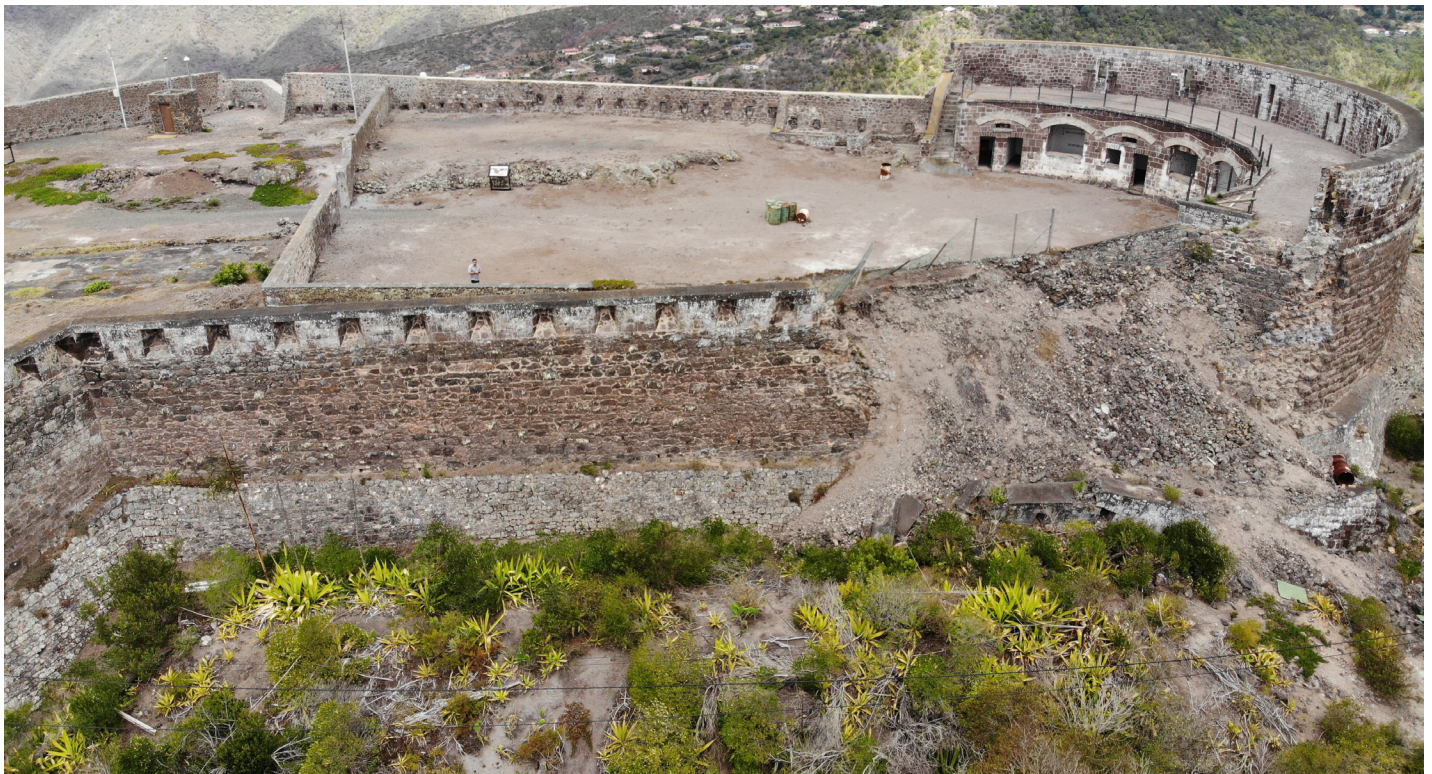
Figure 17: Oblique aerial view of wall collapse from southwest corner of fort with adjoining western wall in view (Image: B. Fortenberry).
