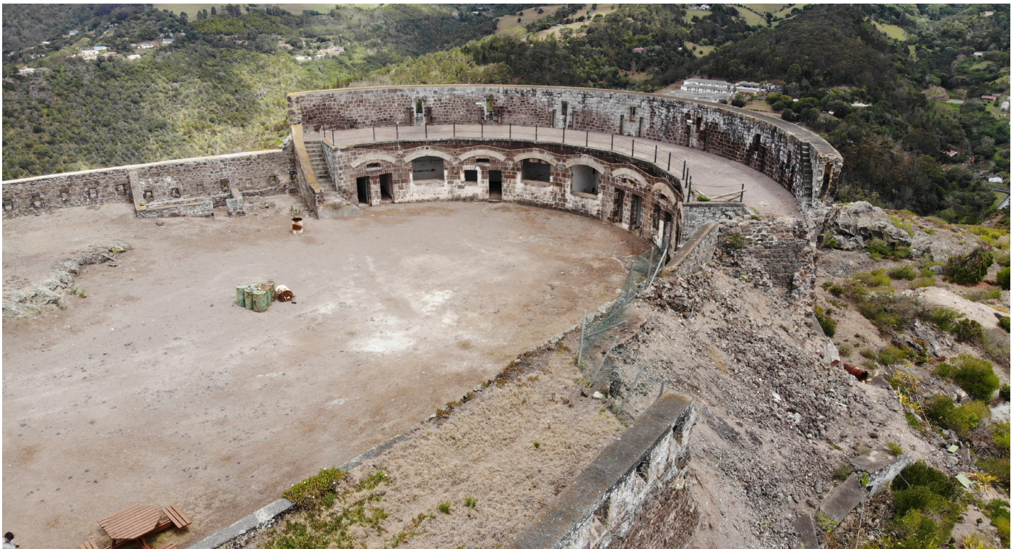
Figure 19: Oblique Aerial view of wall collapse from southwest corner of fort looking southeast (Image: B. Fortenberry).
