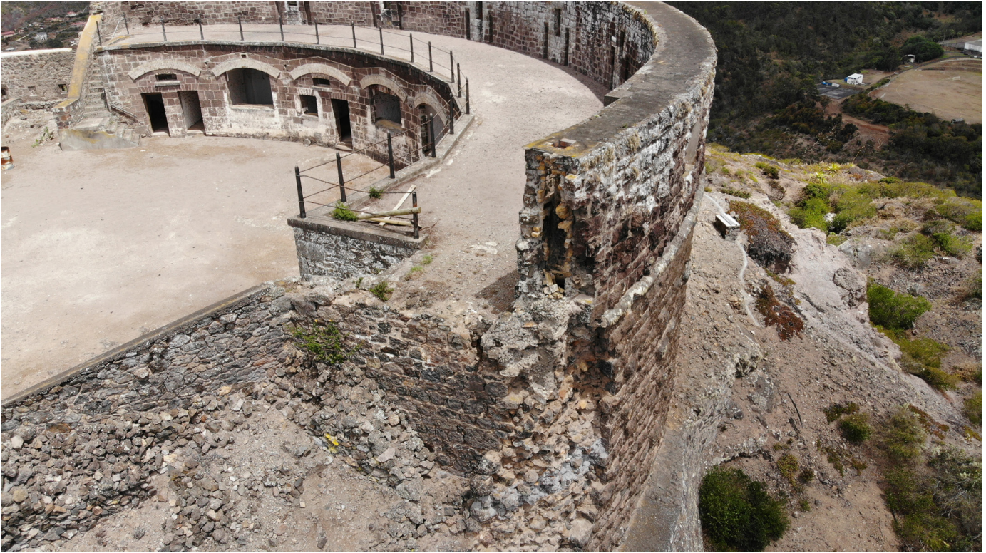
Figure 26: Aerial view of wall collapse from southwest corner with wall section in detail (Image: B. Fortenberry).
