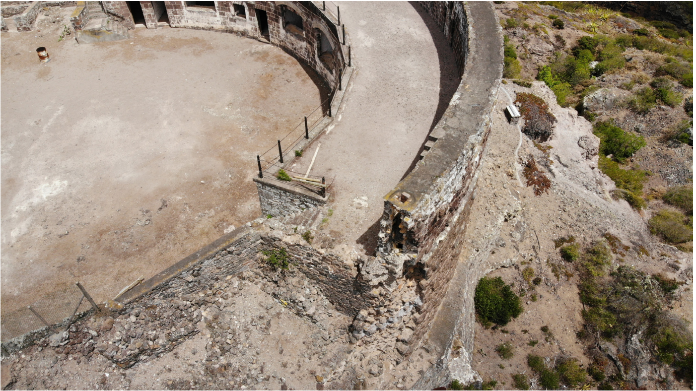
Figure 24: Aerial view of wall collapse from southwest corner with wall section in detail (Image: B. Fortenberry).
