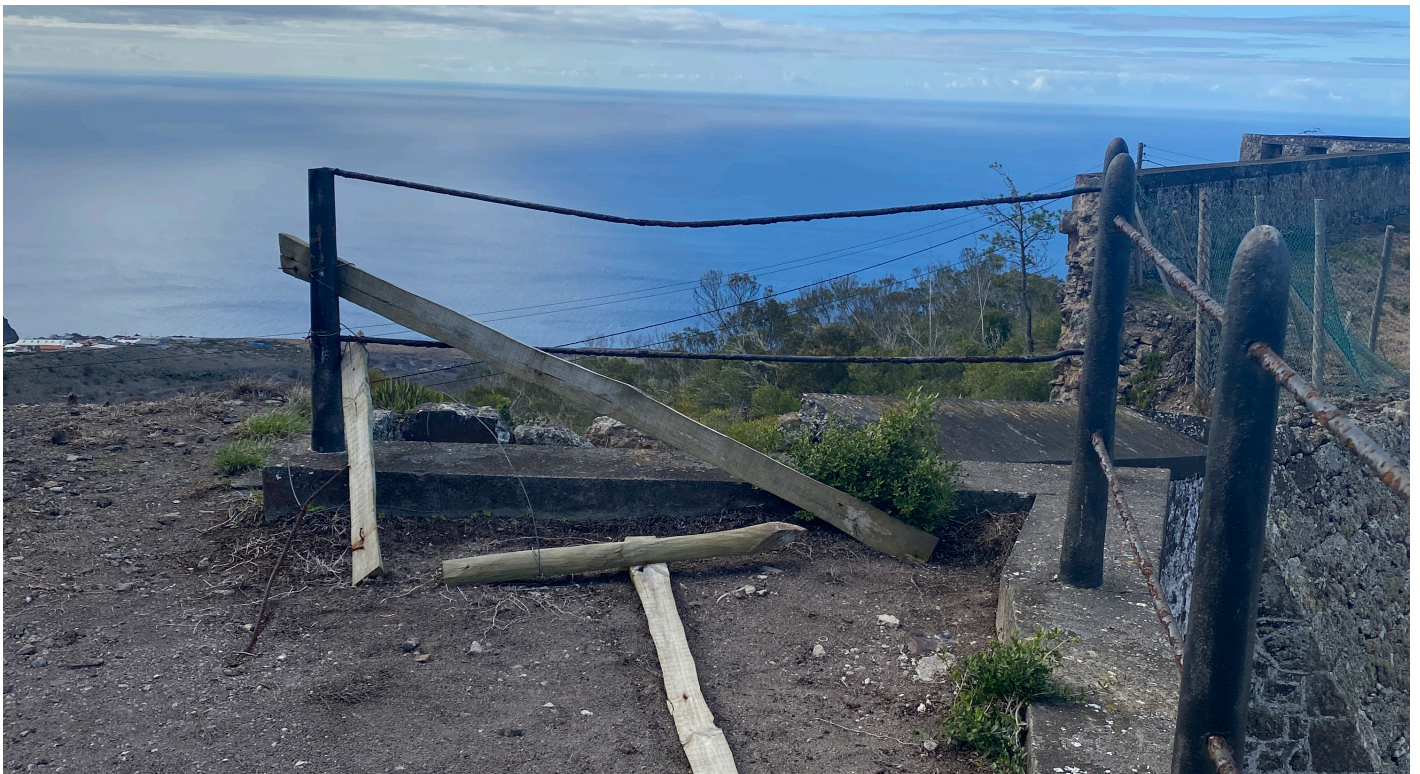
Figure 63: Cast iron pier and guard rail failure on southern firing platform (Image: B. Fortenberry).
