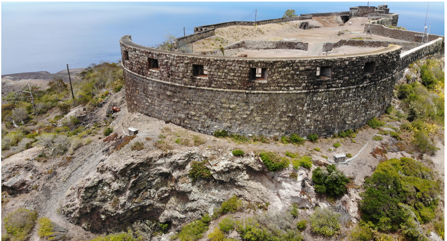
Figure 48: Aerial image of bio-growth on the southern bastion (Image: B. Fortenberry).
