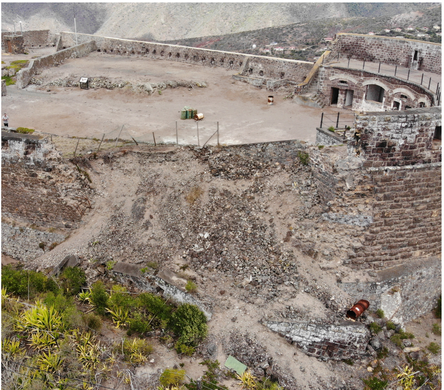
Figure 15: Oblique aerial view of wall collapse from southwest corner of fort (Image: B. Fortenberry).
