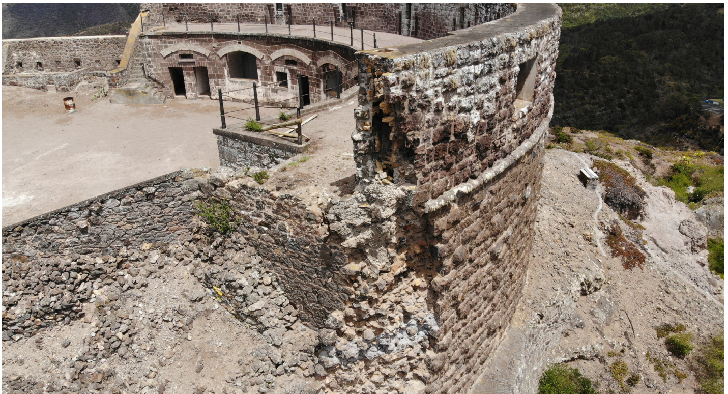
Figure 27: Aerial view of wall collapse from southwest corner with wall section elevation in detail (Image: B. Fortenberry).
