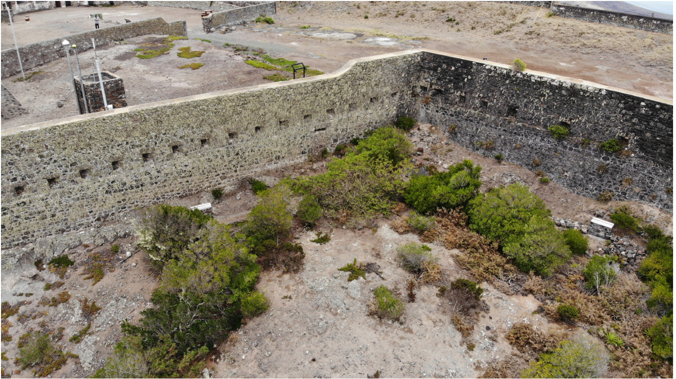
Figure 51: Aerial image of bio-growth on the eastern wall (Image: B. Fortenberry).
