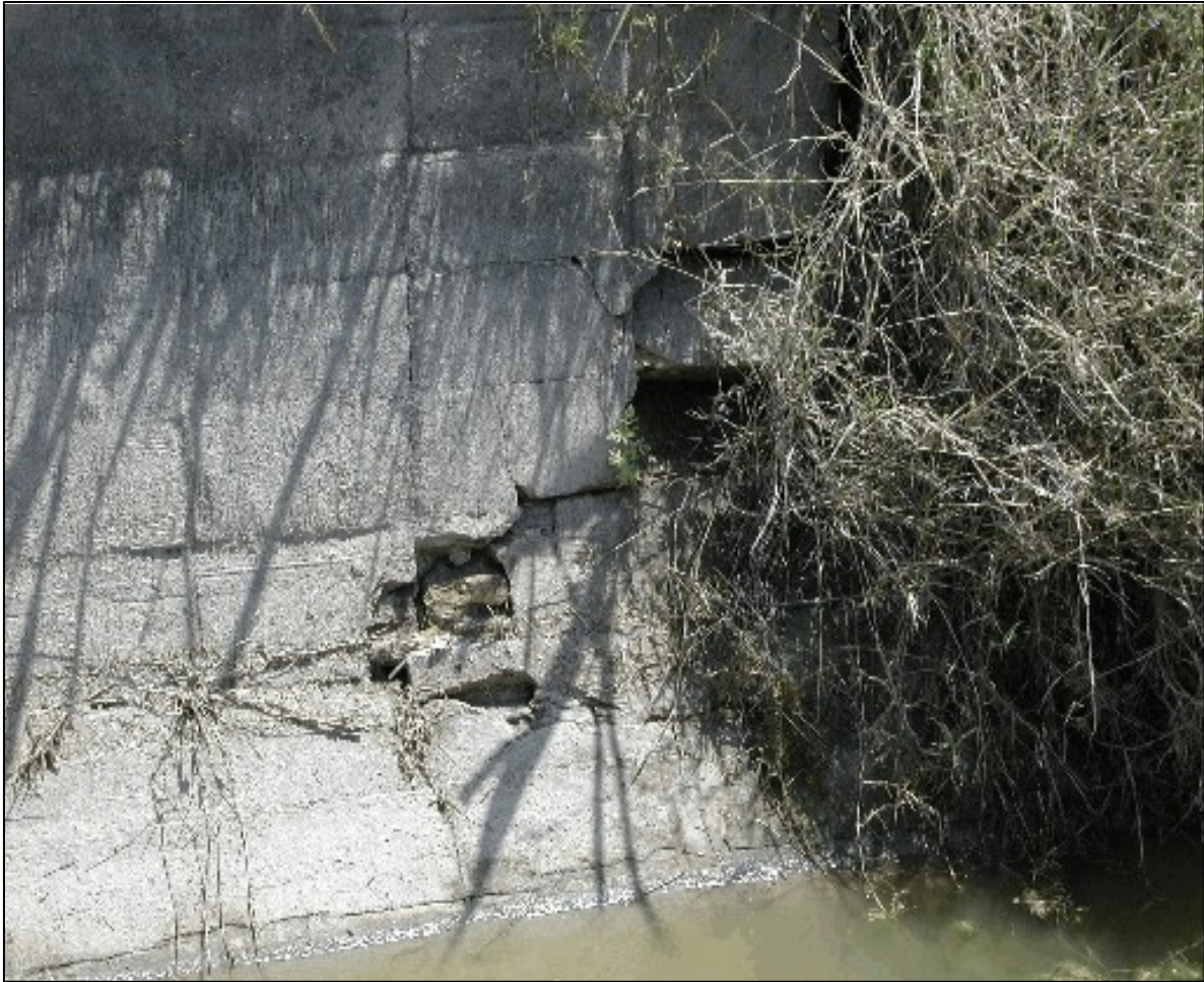
Figure 2. One of six large holes observed in the brick/concrete lining of the south test segment of Canal 6.0.
