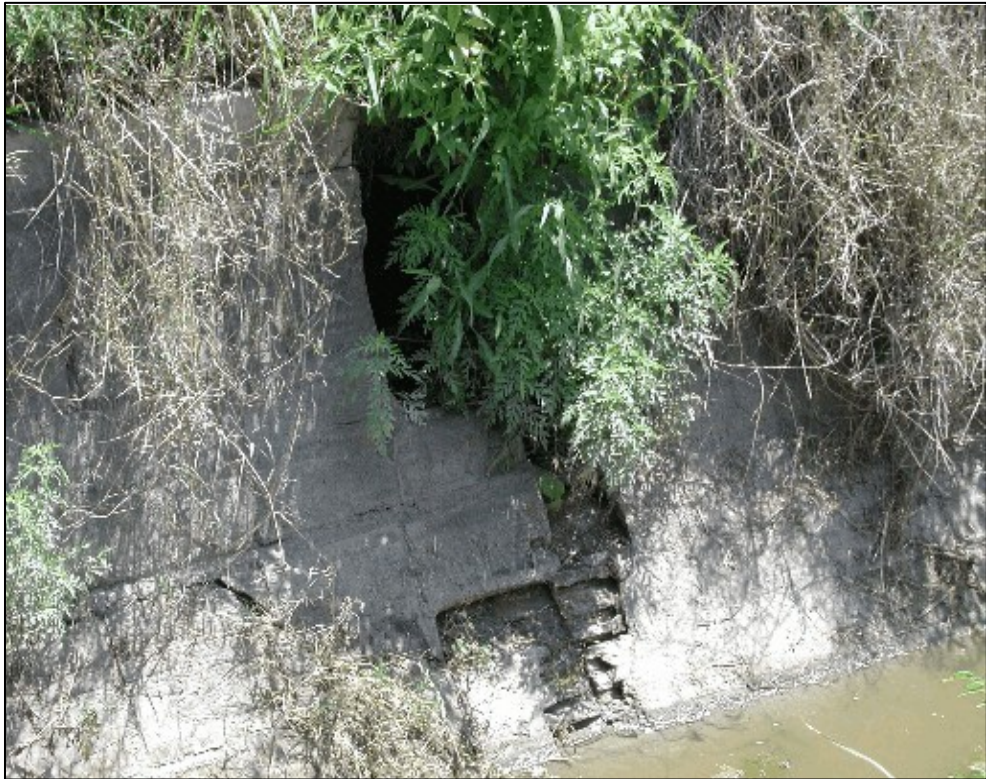
Figure 9. Large hole in the canal lining of Canal 6.0 - South1
