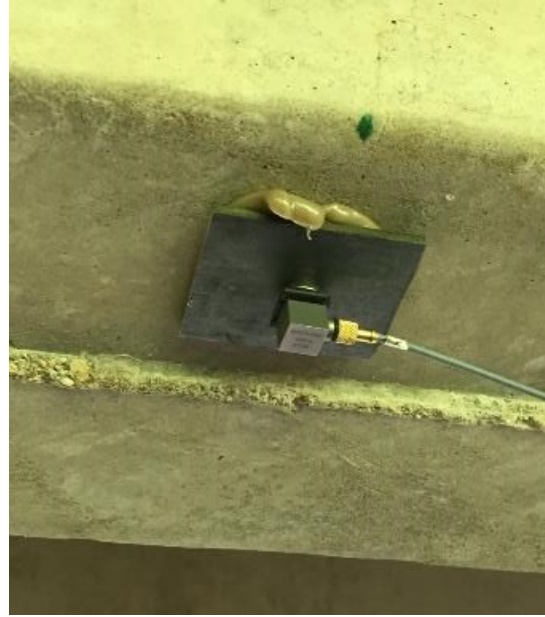
(b) Installed Accelerometer
