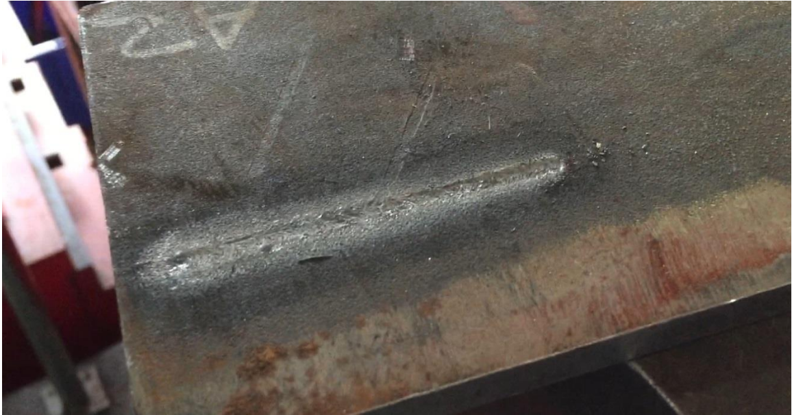
Figure 16: A typical case of damage to backing plate caused by over-penetration of weld.
