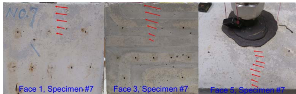
Figure 2.13 Observation of several localized permeation spots/cracks.
