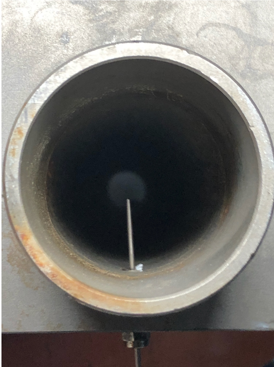
Figure 7.9: Thermocouple placement in riser column of WRCCS facility.
