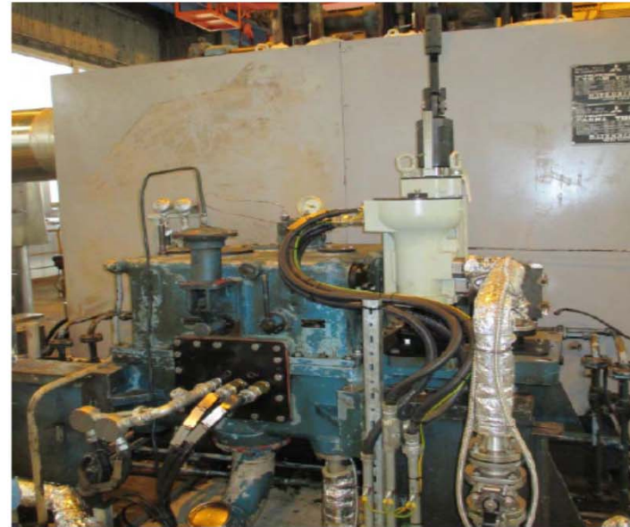
Direct-drive Actuator (After Revamp)
