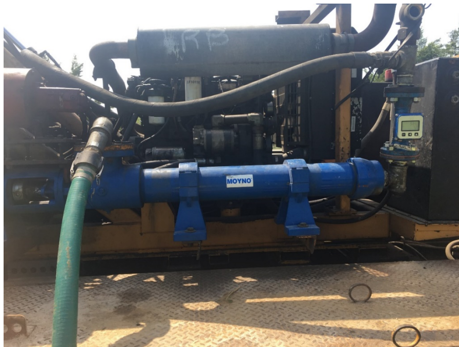
Figure 69. Photograph of the pump and the in-line flowmeter assembly on the drill rig
