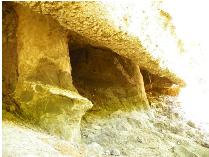
Figure 51- Voids under the left abutment concrete riprap of CR 309 over Rocky Creek
