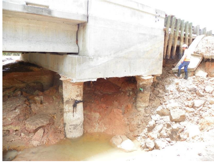
Figure 53- Right abutment failure at SH 105 over Rock Creek
