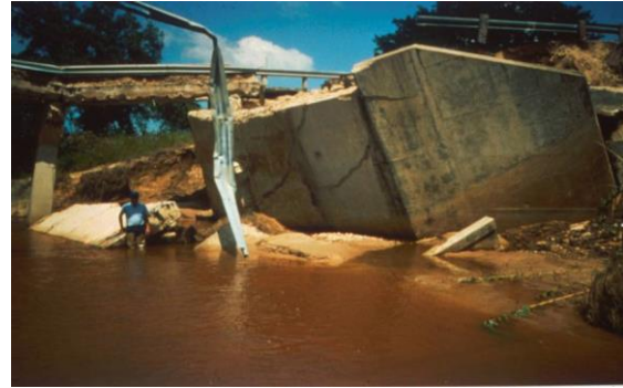
Figure 58- Abutment foundation failure by horizontal loading
