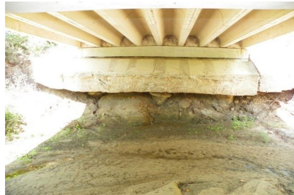
Figure 60- Erosion of the embankment soil
