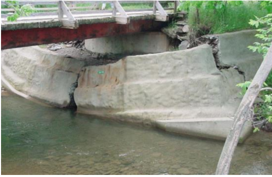
Figure 57- Abutment foundation failure by vertical loading
