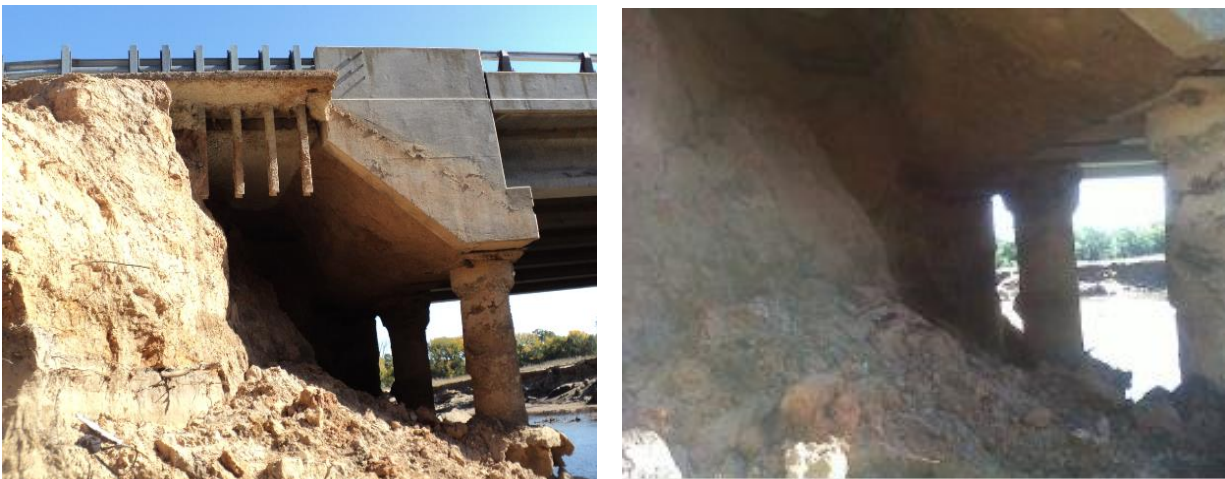
Figure 48- Left abutment failure at FM 937 over Montgomery Creek
