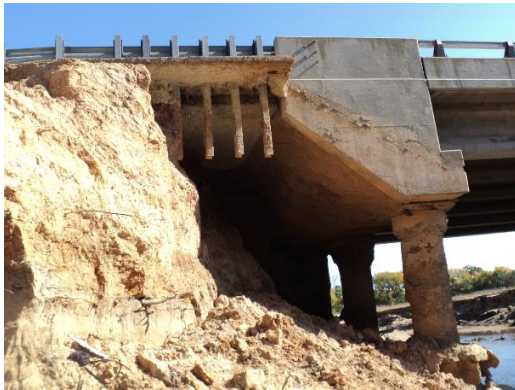
Figure 59- Slope stability failure of the abutment embankment
