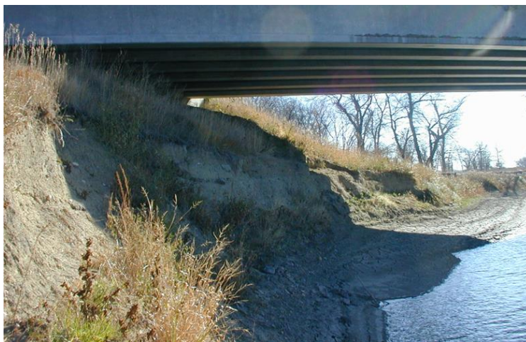
Figure 45- Scour at the left abutment of SR 37 over James River during the flood
