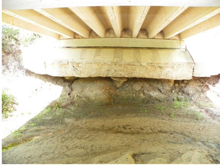
Figure 50- Scour at the left abutment of CR 309 over Rocky Creek
