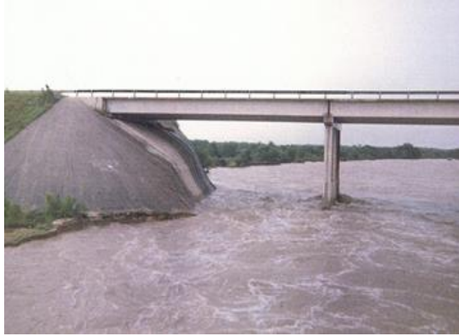
Figure 54- Right abutment failure at US 90 over Nueces River
