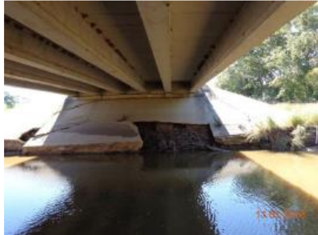
Figure 49- Damaged concrete riprap at the right abutment of FM 937 over Montgomery Creek
