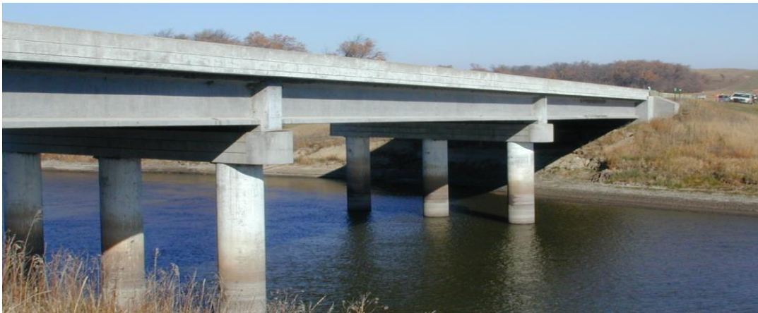
Figure 43- SR 37 over James River after the flood—looking at the left abutment from the downstream
