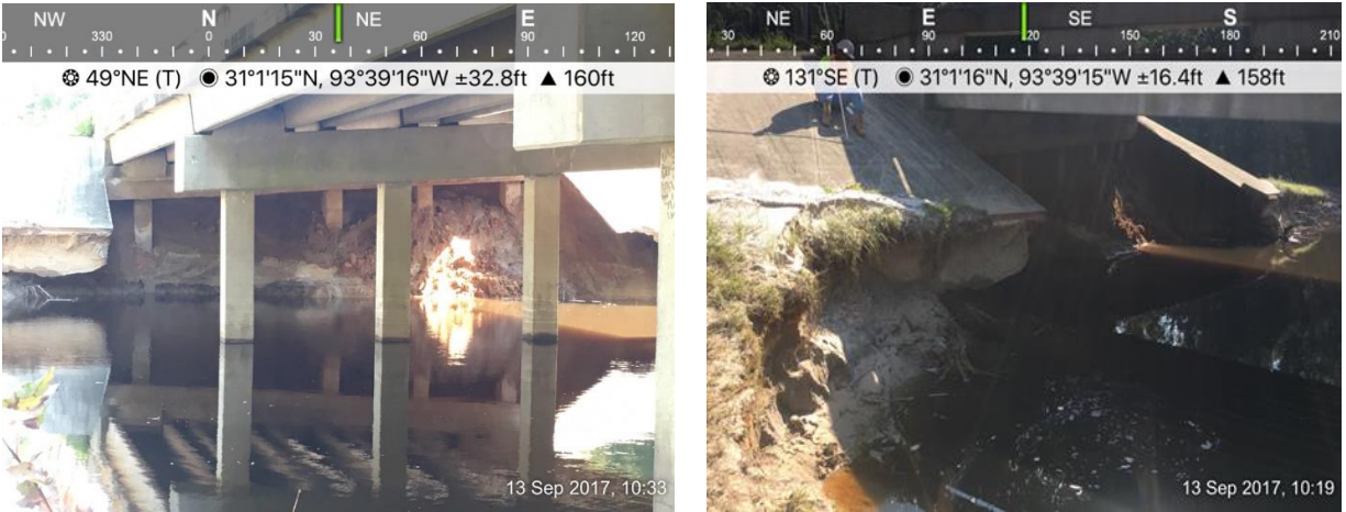
Figure 46- Left abutment failure at FM 692 over McGraw Creek
