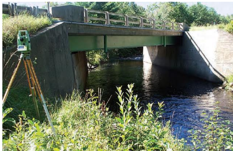
Figure 39- Typical abutment configuration and location at the studied bridge sites in Maine (reprinted from Hodgkins 2008)
