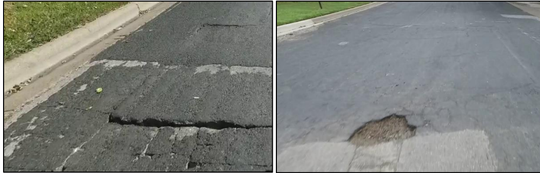
Figure 13. Instances of Road Anomalies: Deep Crack and Pothole
