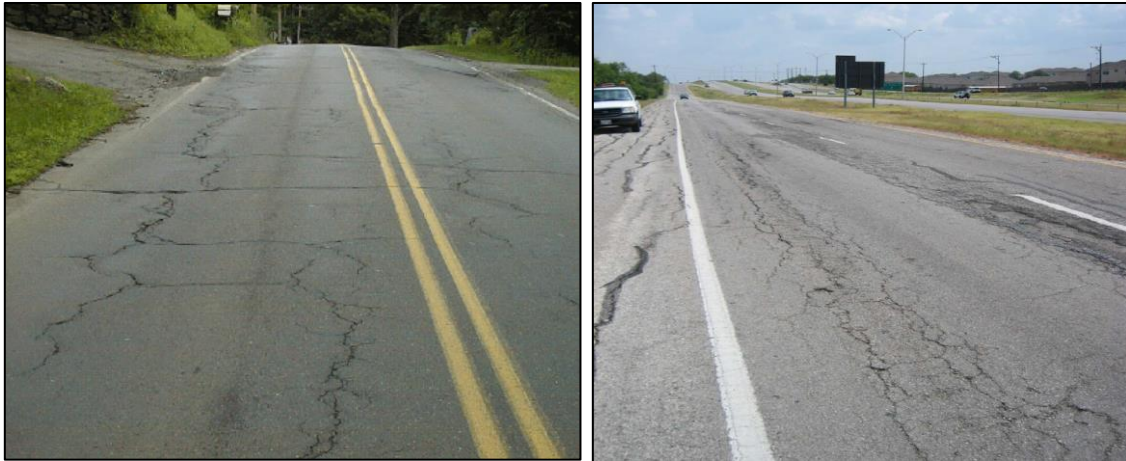
Figure 3. Instance of Block Cracking and Alligator Cracking. Reprinted from [7].
