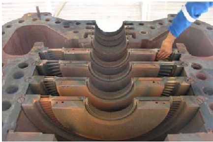
Figure 5 - Unreliable Stage #5 Original Diaphragm: Vanes at Joint can be Shaken by Hand
