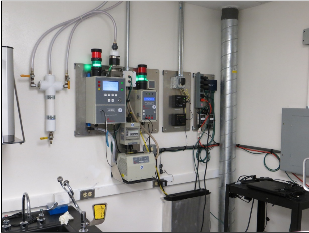
Figure 38. The facility radiation monitors are shown. On the left is the iCAM model continuous particulate air monitor. On the right is the G64 model area gamma alarm.
