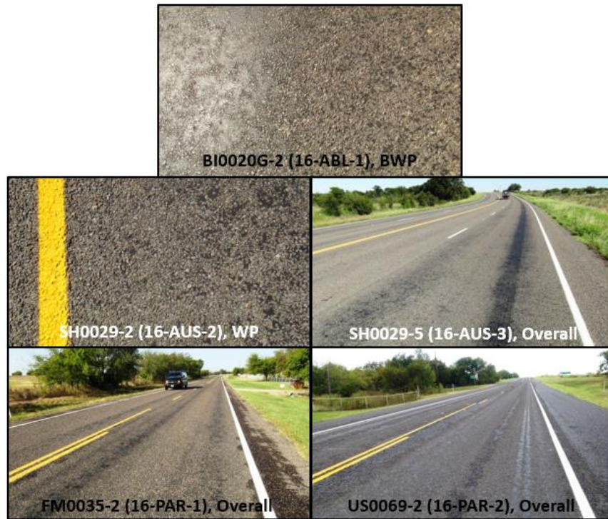
Figure 26. Pictures Depicting Flushing in HSs That Exhibited High ED Post-Construction.
