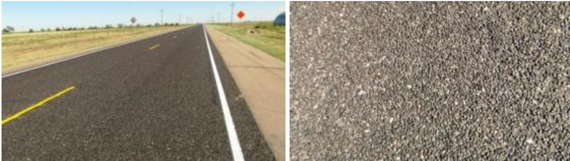
Figure 28. Example of Adequate Performance—16-AMA-1, Post First Winter.
