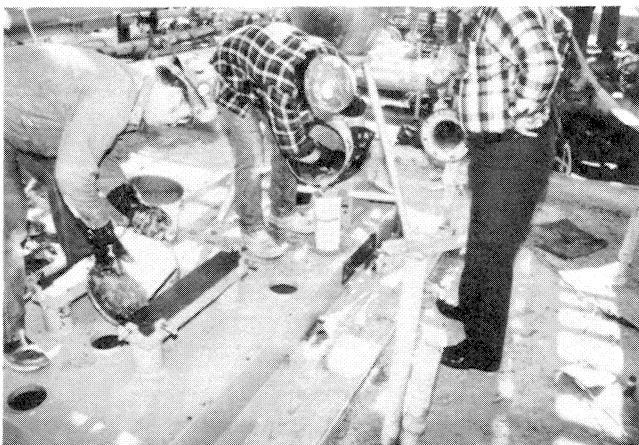
Figure 22. The Resin Containers Are Used to Place Grout in the Center Baseplate Grout Holes.
