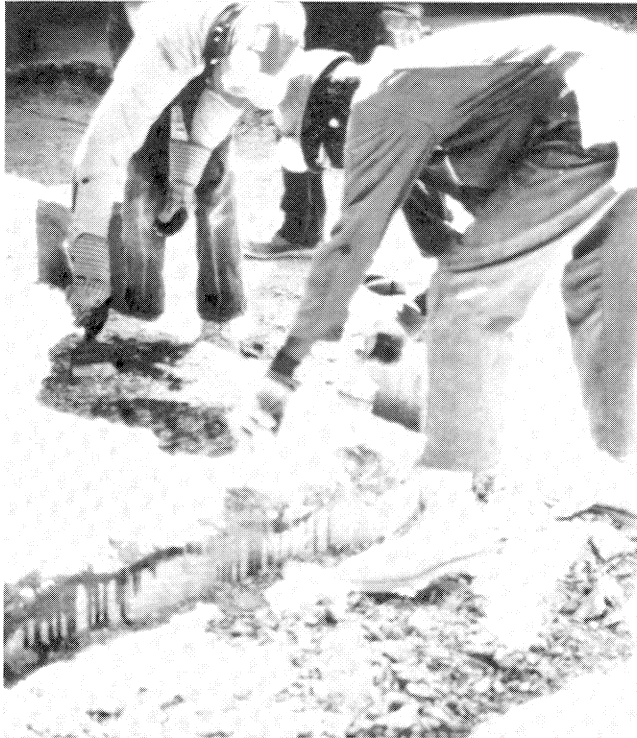
Figure 11. Coat the Clean, Dry, Chipped Concrete with a Coating of Unfilled (Without Aggregate) Epoxy Grout.
