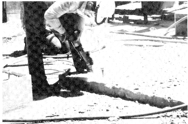
Figure 9. All Laitance Must Be Chipped Off the Surface of the Foundation to Expose the Aggregate.
