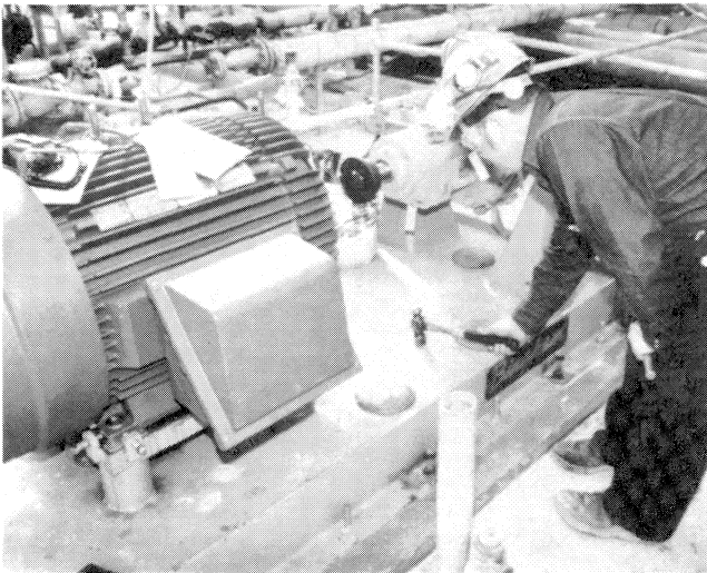
Figure 30. A Hammer Was Used to Test the Baseplate Grout Job for Voids.
