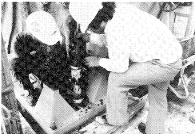
Figure 26. Once the Grout Cylinder was Filled, the Grout Pump Piston Was Installed and Pressed Down.
