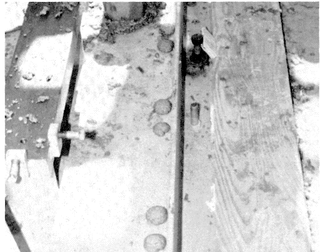
Figure 24. Notice the Air and Grout Flowing from the Baseplate Vent Holes. A vent hold was drilled on each side of the cross braces.
