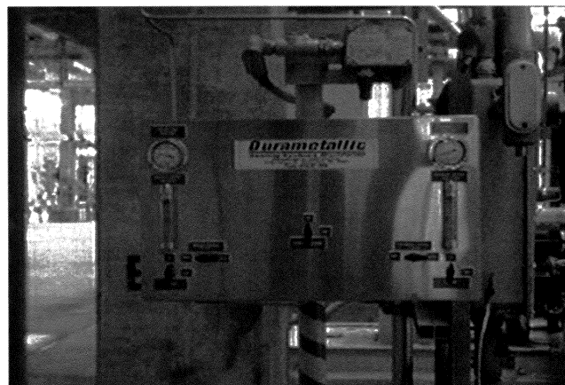
Figure 9. Dual Nonpressurized Seal Control Panel.
