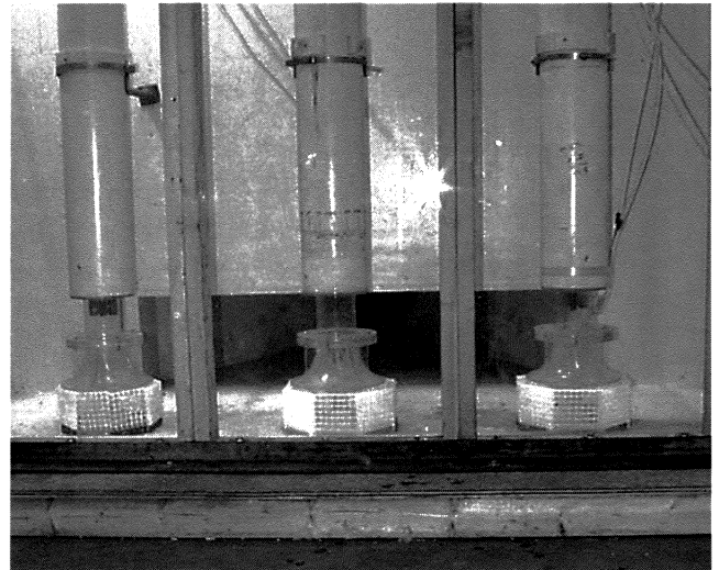
Figure 18. Mod 2 Installed on Pumps.
