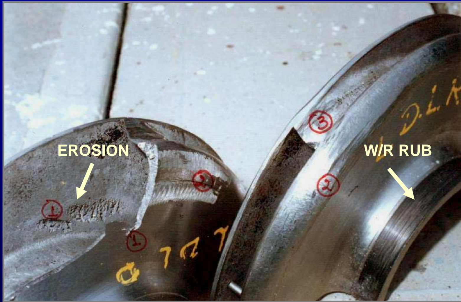
SEVERE IMPELLER FAILURE - 1992
