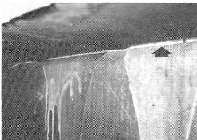
Figure 6. Bleed of Excess Epoxy from Beneath a Steel Plate Stiffener which was Field Installed. Because of the Large Gap, a "Thickened" Epoxy was used in Order to Maintain Capillary Contact Between the Two Surfaces.
