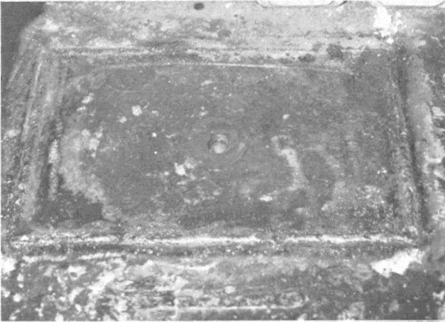
Figure 13. A Typical Vent Hole is Shown in the Access Plate After It has been Welded in Place.
