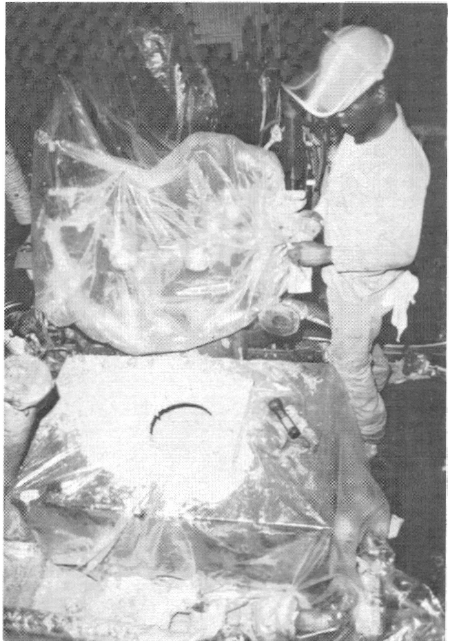
Figure 11. The Gear Box Support Cavity is Being Filled with Successive Pours of Epoxy Mortar to Unload the Box and Gain Rigidity.
