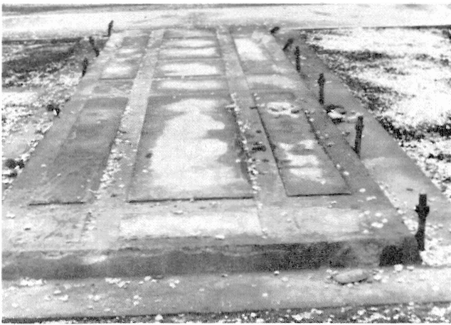
Figure 2. A Properly Grouted Platform which Later was Removed from its Concrete Pad. Note that 100% Contact had been Obtained by the Grout on All Longitudinal and Transverse Supporting Beams.
